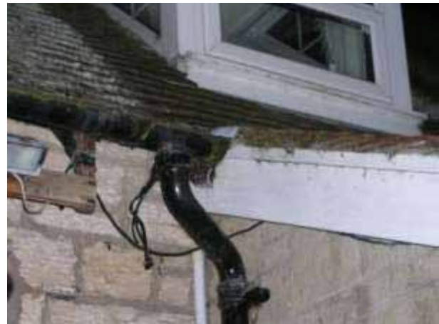
Gap above the gutter adjacent to the lean-to used by bats.
