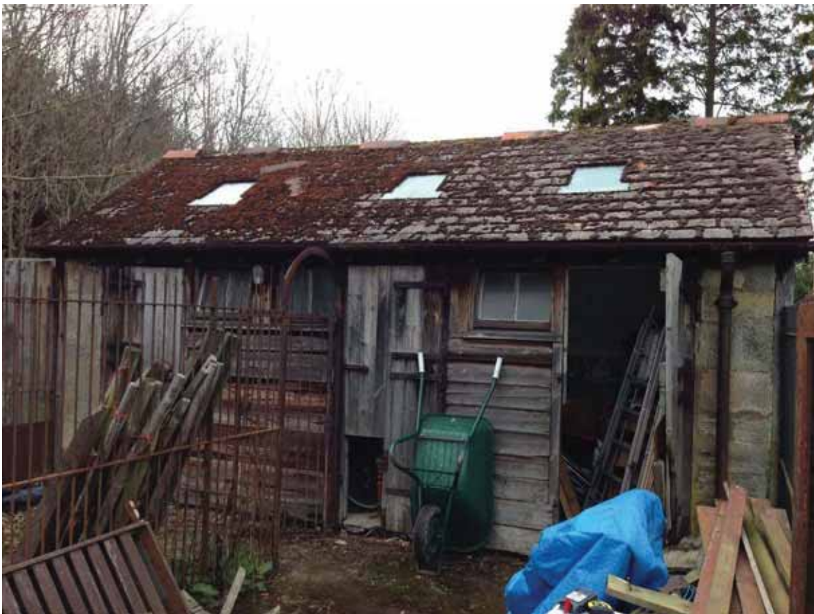
South elevation showing moss to the roof and the lack of decoration to the timber elements and defective boarding.
