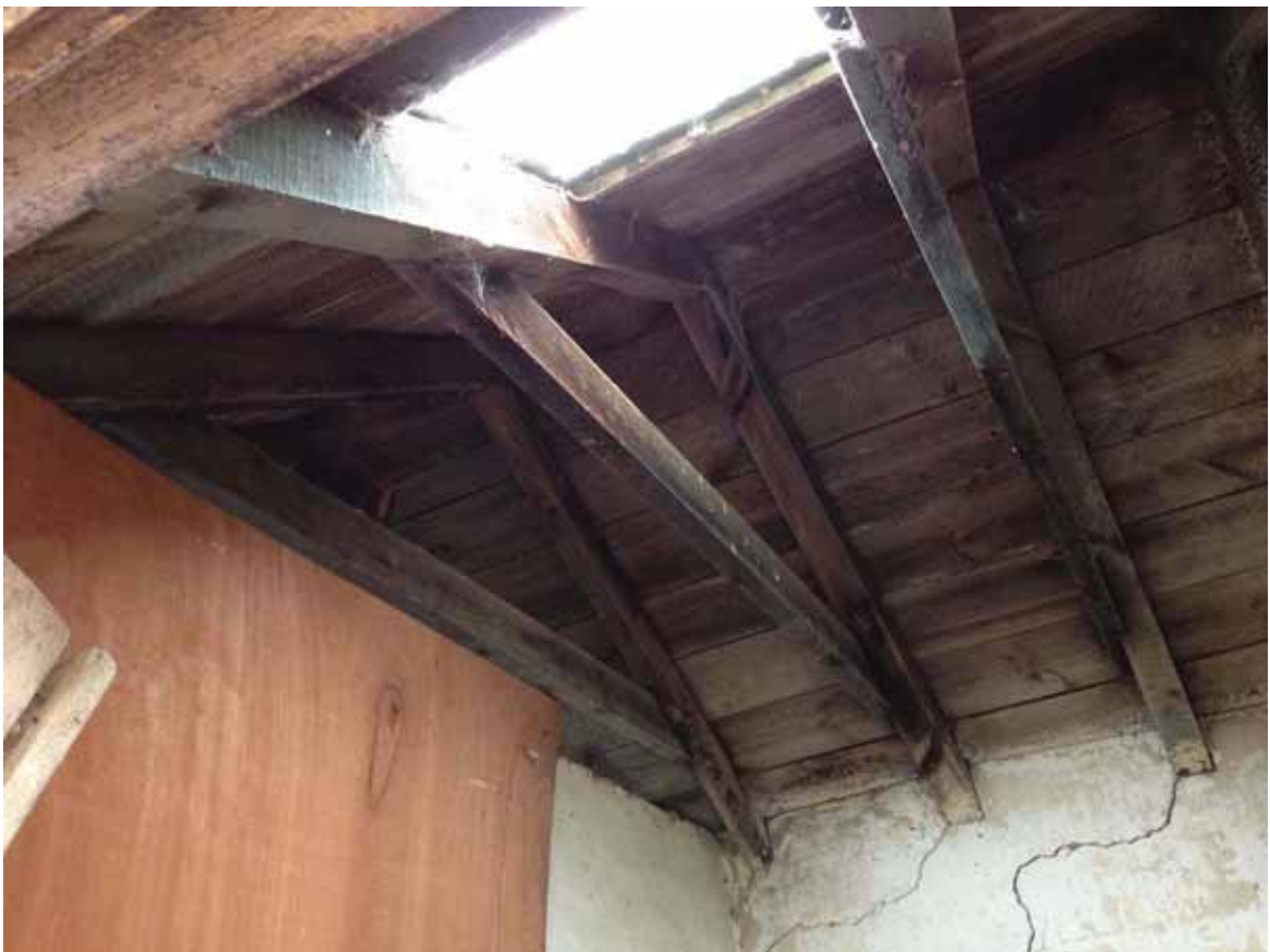
Internal roof structure showing the good condition of the timbers and sarking board. The cracking shown below the timbers was to the plaster finish only and was checked from both sides.
