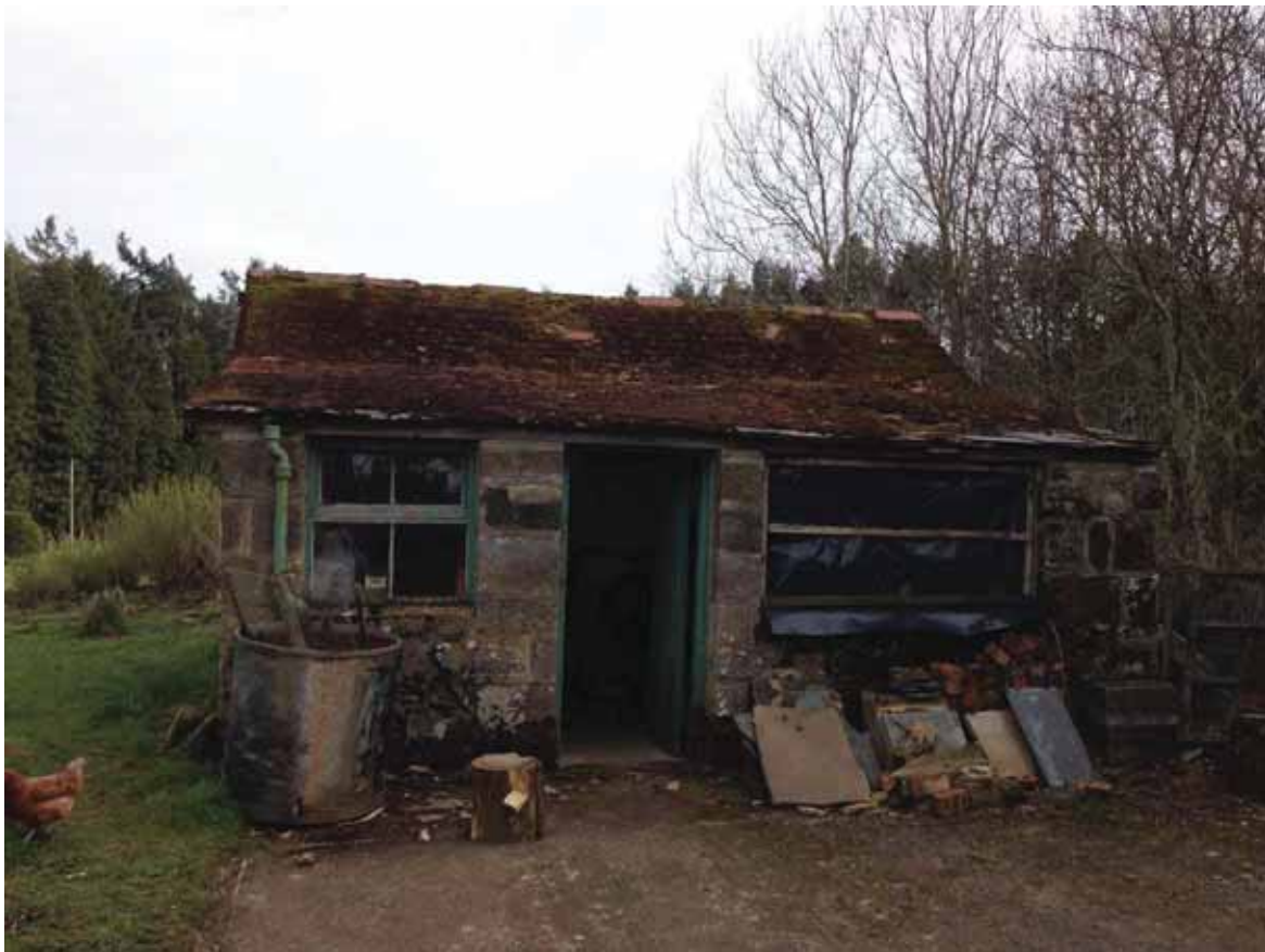
North elevation showing a heavy moss covering to the roof along with defective and missing timber elements to the openings.
