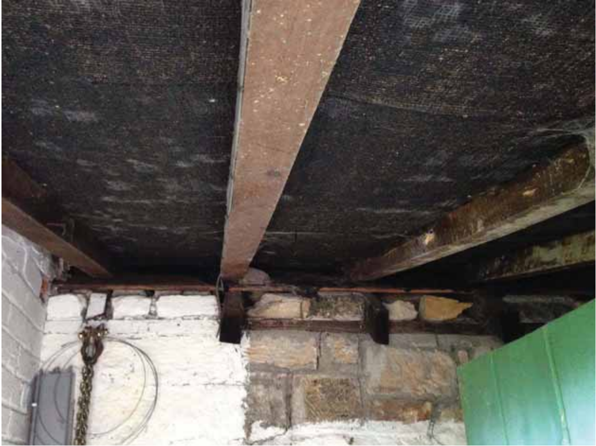
Photo of the lean-to roof and the existing felt underlay with the timbers in good condition
