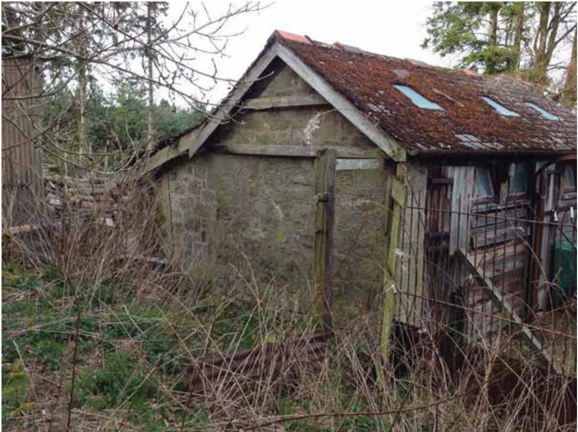
West elevation showing defective barge and gable timbers, but good condition of stonework with signs of remedial pointing to the lean-to section.
