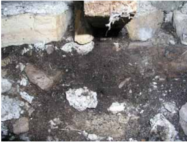
Photo showing disintegrated bat droppings beneath coping stones. If examined carefully, in the black dust exoskeletons of insects can be seen shining.
