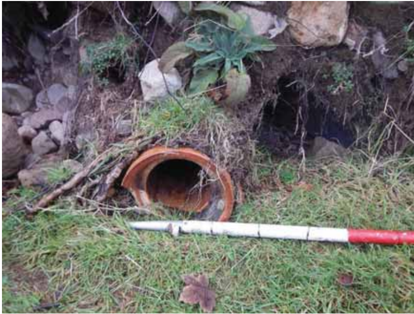
Photograph 2: A disused 90mm diameter main feed pipe of the former surface water abstraction
