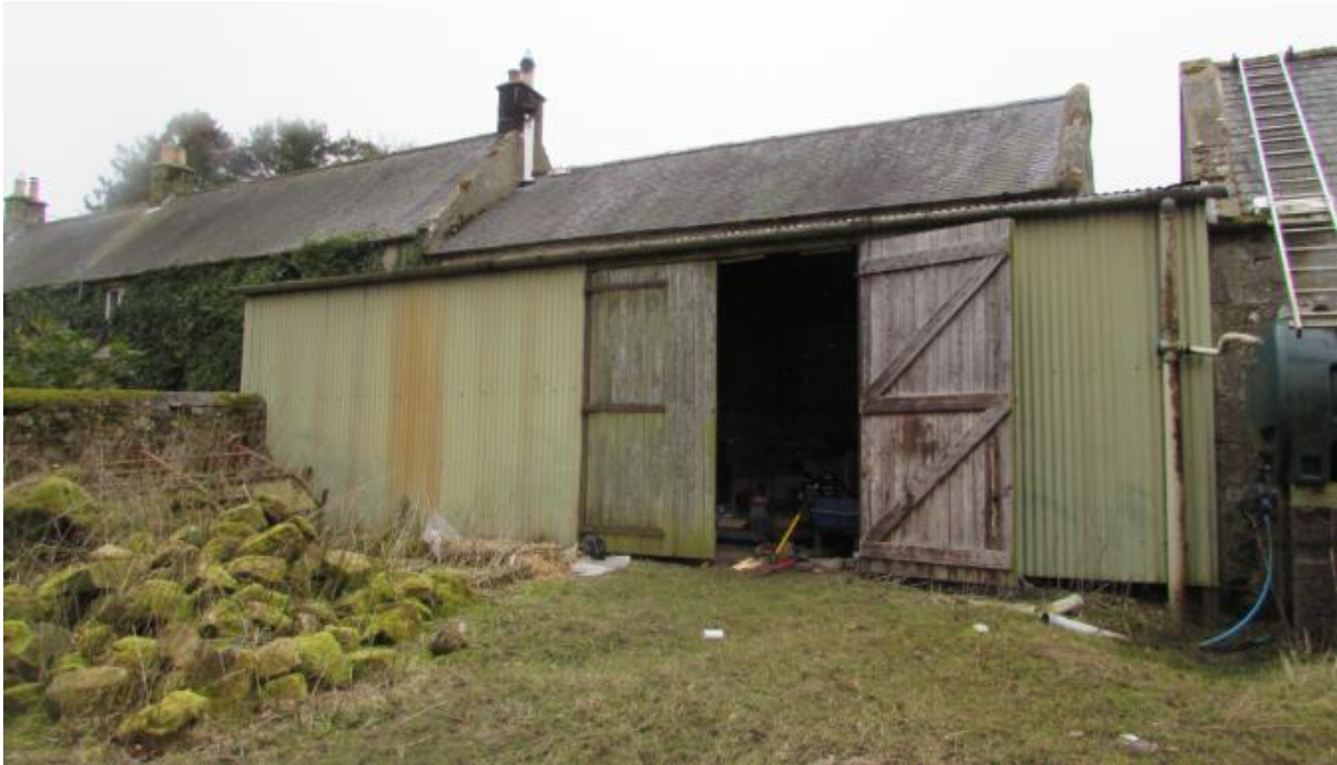
Front (eastern) elevation of existing lean-to shed, with existing outbuildings to the rear and right. Farmhouse to the left, beyond stone garden wall. The proposed extension would replace the shed in this location with non-opening glazing to the facing elevation.
