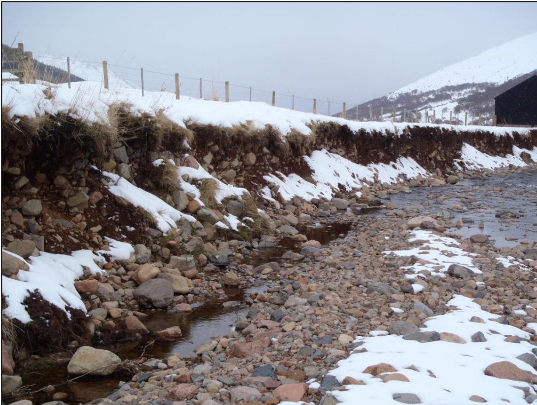
Figure 2.5. Bank erosion within the upper half of the survey reach.
