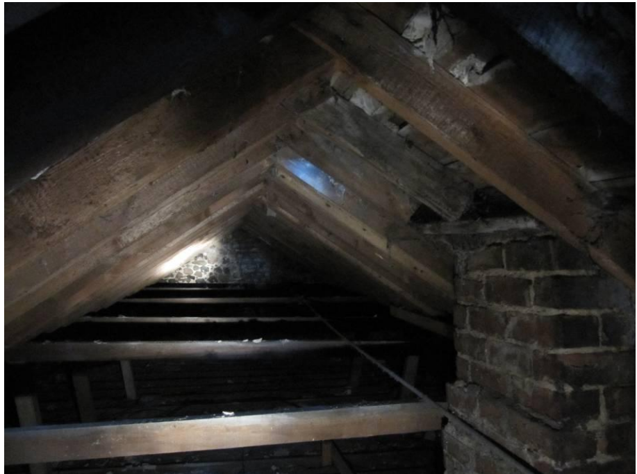
Photo 4. Interior of bungalow (building 1) roof void. Note light entering through gap created by missing roof slate.
