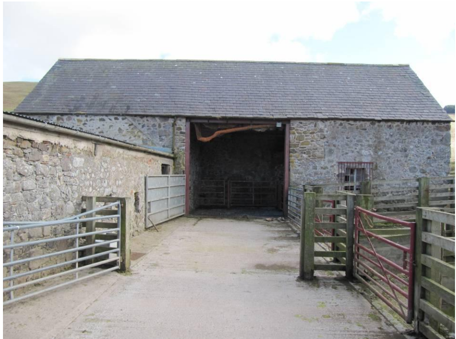
Photo 6. Traditional two-storey and store barns (buildings 2a and 2b), viewed from the north-west.
