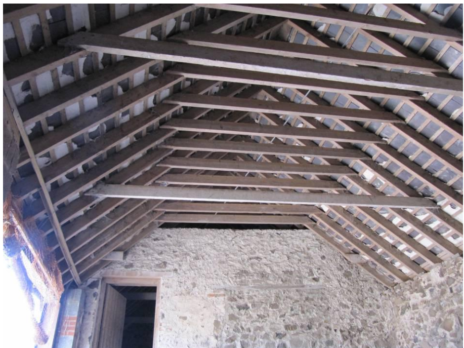
Photo 8. Roof void of traditional two-storey barn (building 2a) with access to first-floor hay-loft.
