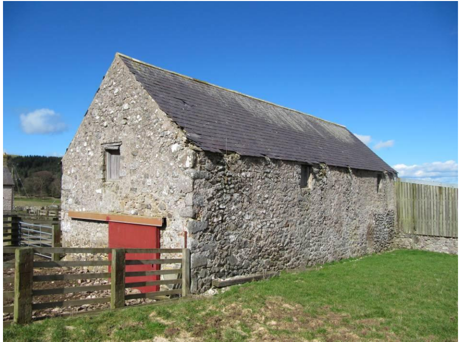
Photo 7. Traditional two-storey barn (building 2a), viewed from the south. Note missing roof slates and missing mortar with potential crevices in walls.
