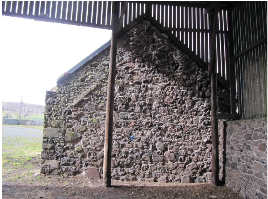
Photo 12. Gable of traditional stall and store (building 2d), viewed from the south-east. Note missing mortar and potential crevices in wall.
