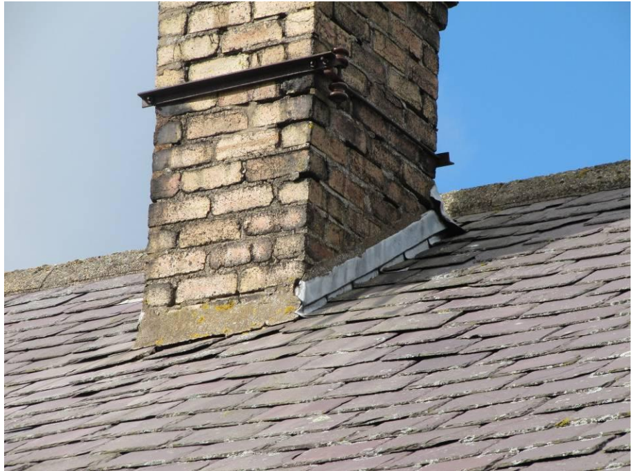
Photo 3. Chimney and surrounding roof on bungalow (building 1). Note potential crevice behind poorly fitted lead flashing.
