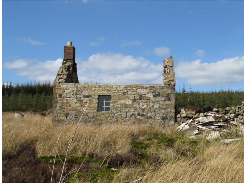
Closer view of south elevation of bothy and rubble resulting from removal of previous roof
