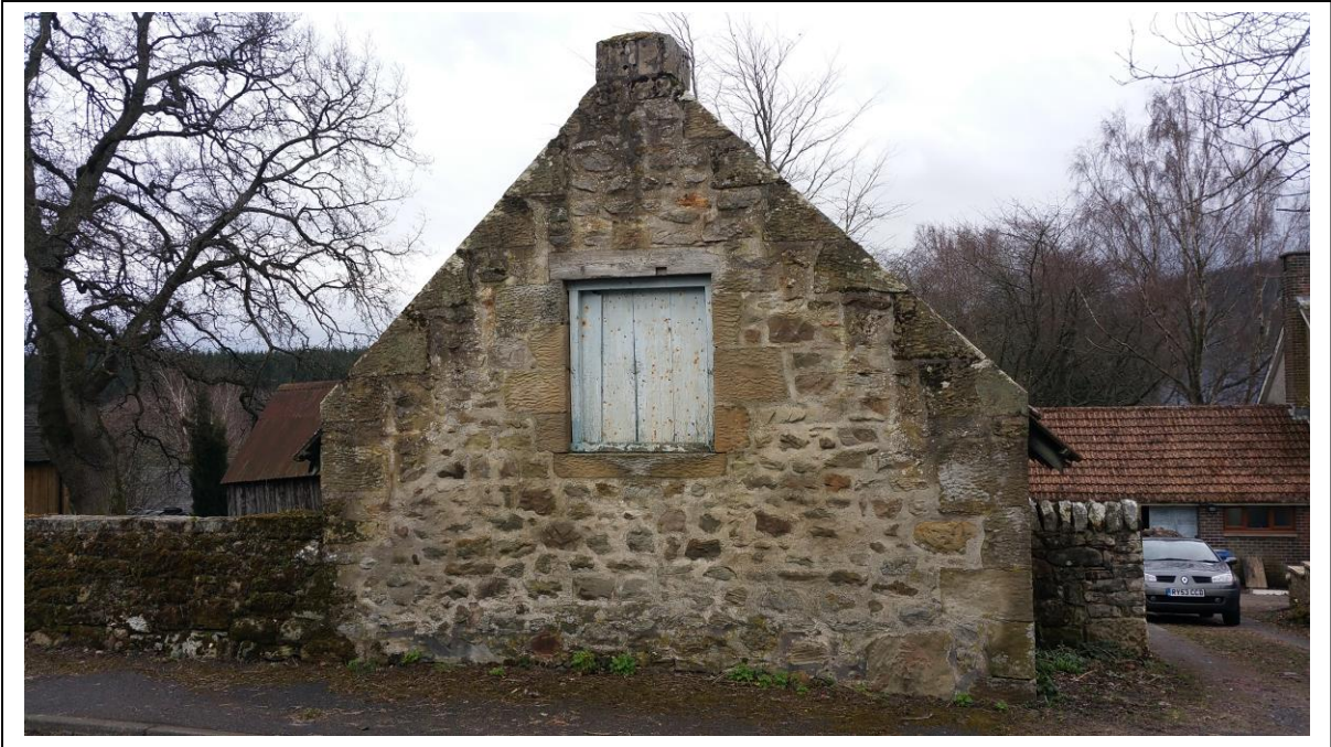
Northern elevation – with boarded window
