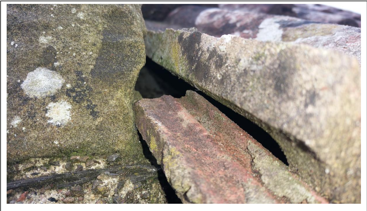
South west corner roof section with slipped tiles
