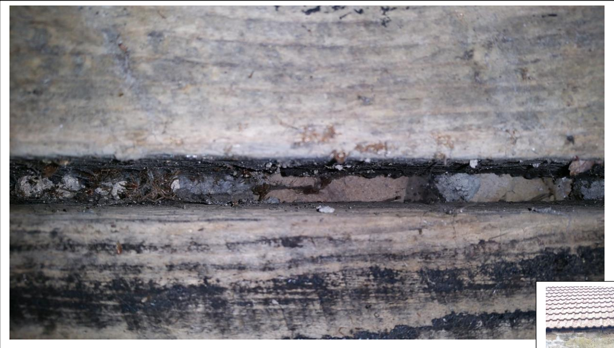
Gap above the doorframe
