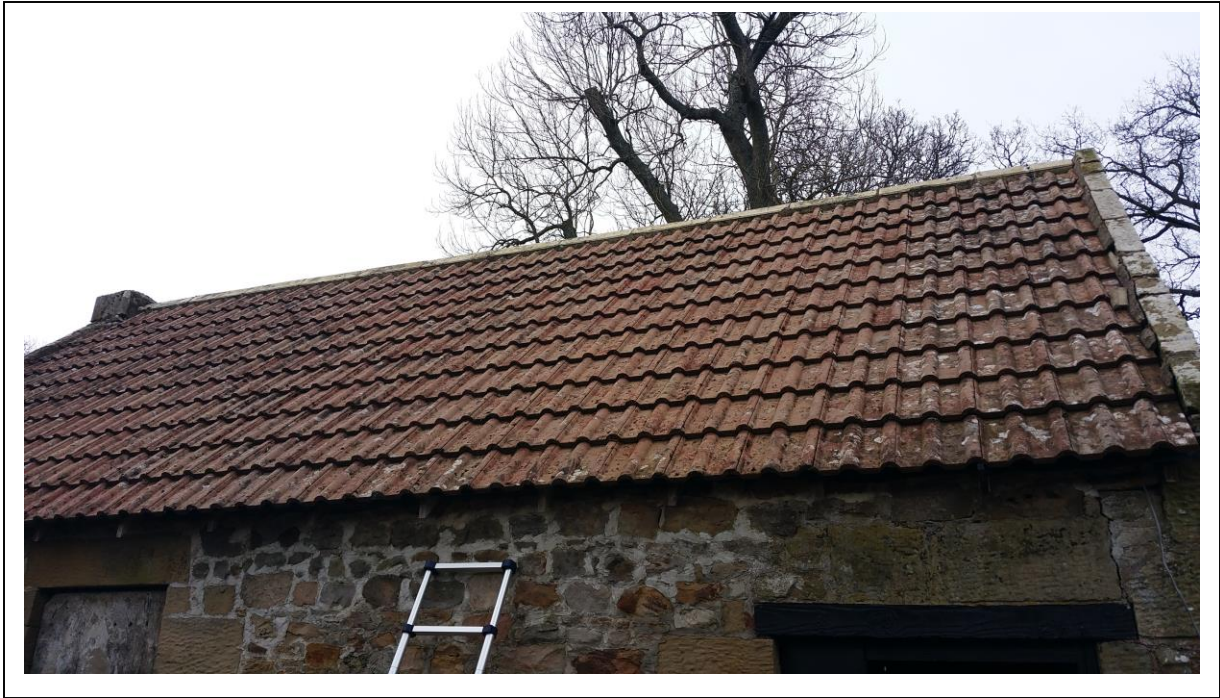
Roof Section – with gaps to the mortar to the southern gable end
