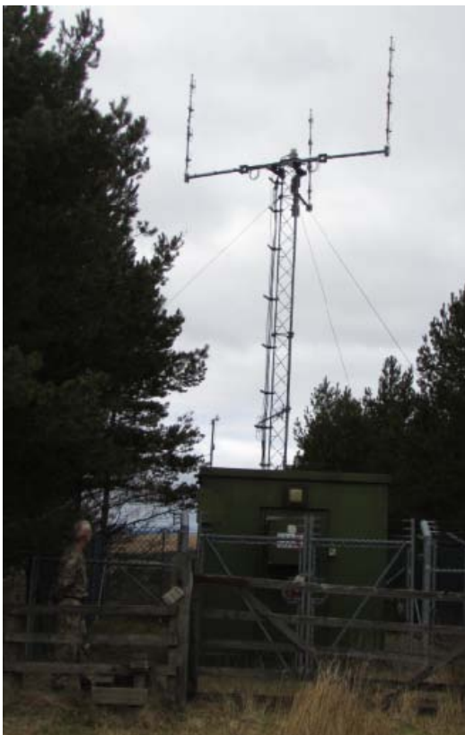
Left: Photograph of existing antenna
