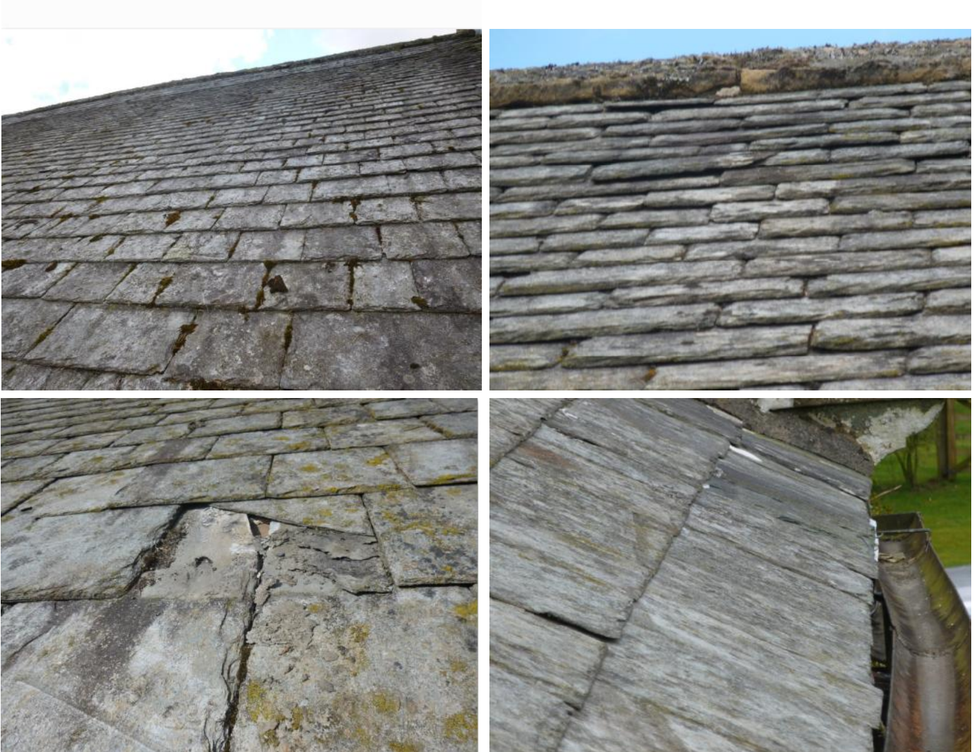
Clockwise from top left: Condition of existing roof; evidence of displaced slates and poor condition of ridge tiles; evidence of cracked and delaminated slates; some existing RWGs of poor condition
