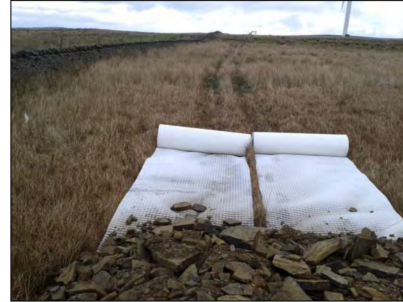
Plate 13: semi-permeable geotextile layer
