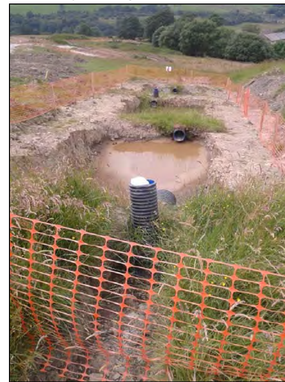
Plate 5: Typical lagoon and flocculent station
