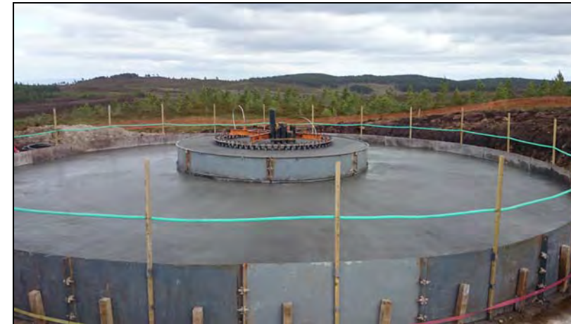
Plate 10: Typical wooden shuttering – to be deployed around the turbine foundations during concrete pours
