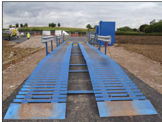
Plate 9: Example of a dry ramp wheel wash facility
