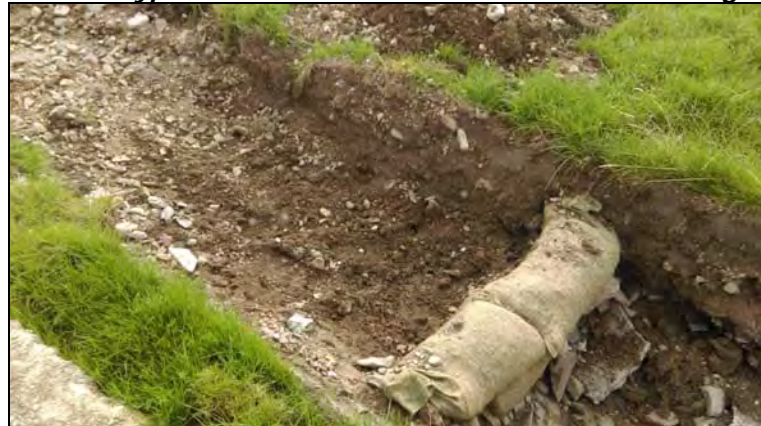
Plate 4: Typical check dams - to be installed in drainage ditches adjacent to the access track
