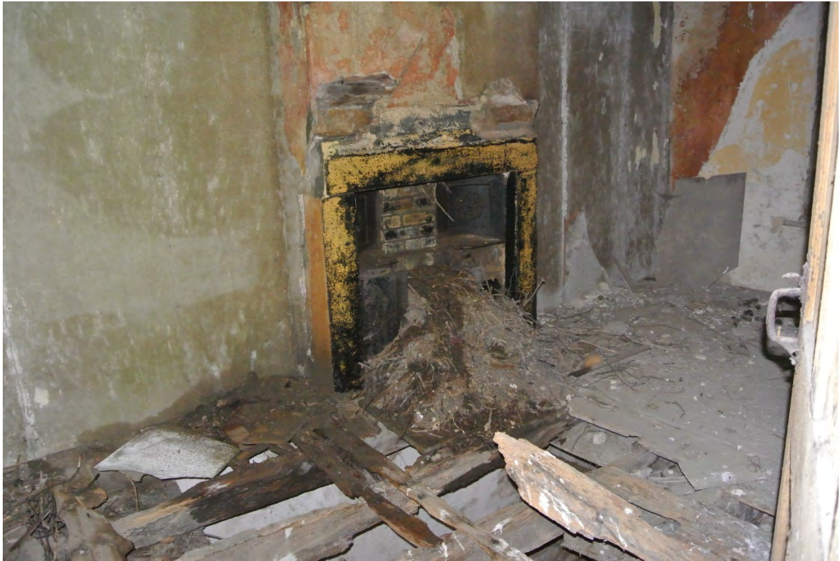
Internal view of East gable at first floor showing fireplace to be overhauled, fibre cement dry lining (ACM), rotten floor etc..
