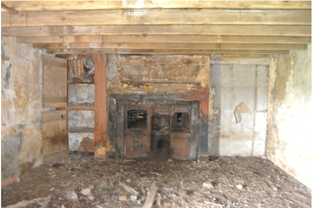
Internal view of West gable at ground floor showing range to be removed, fibre cement dry lining (ACM) to RH side of range and cupboard to LH side of range to be removed.
