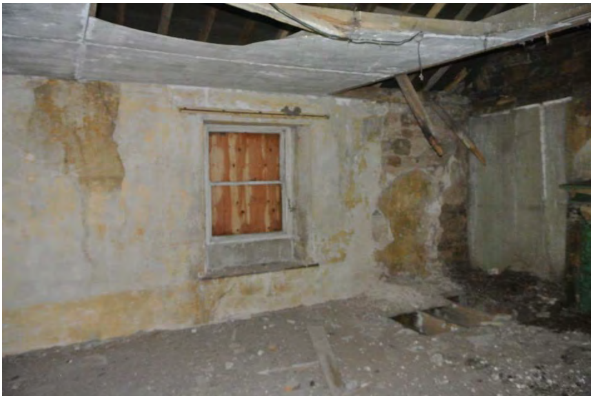
View of South wall in area 6 showing window and fibre cement dry lining / ceiling
