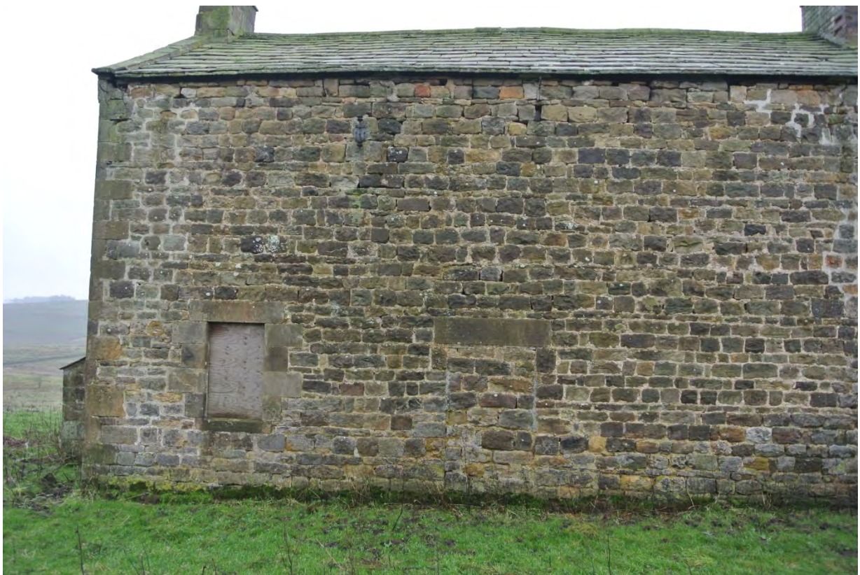
Existing North Elevation showing door to be reopened and location for Bedroom 3 window
