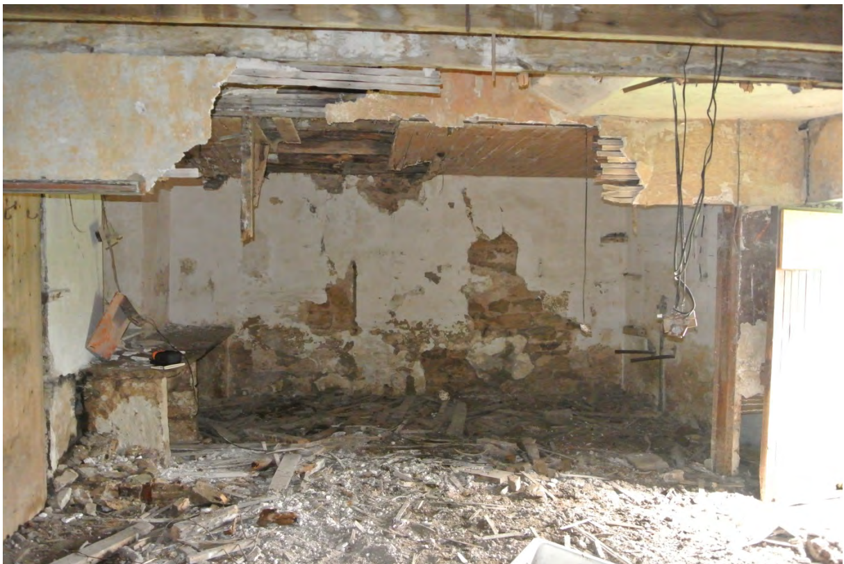
Internal view of East gable at ground floor showing stone shelf at LH side and remnants of partitions
