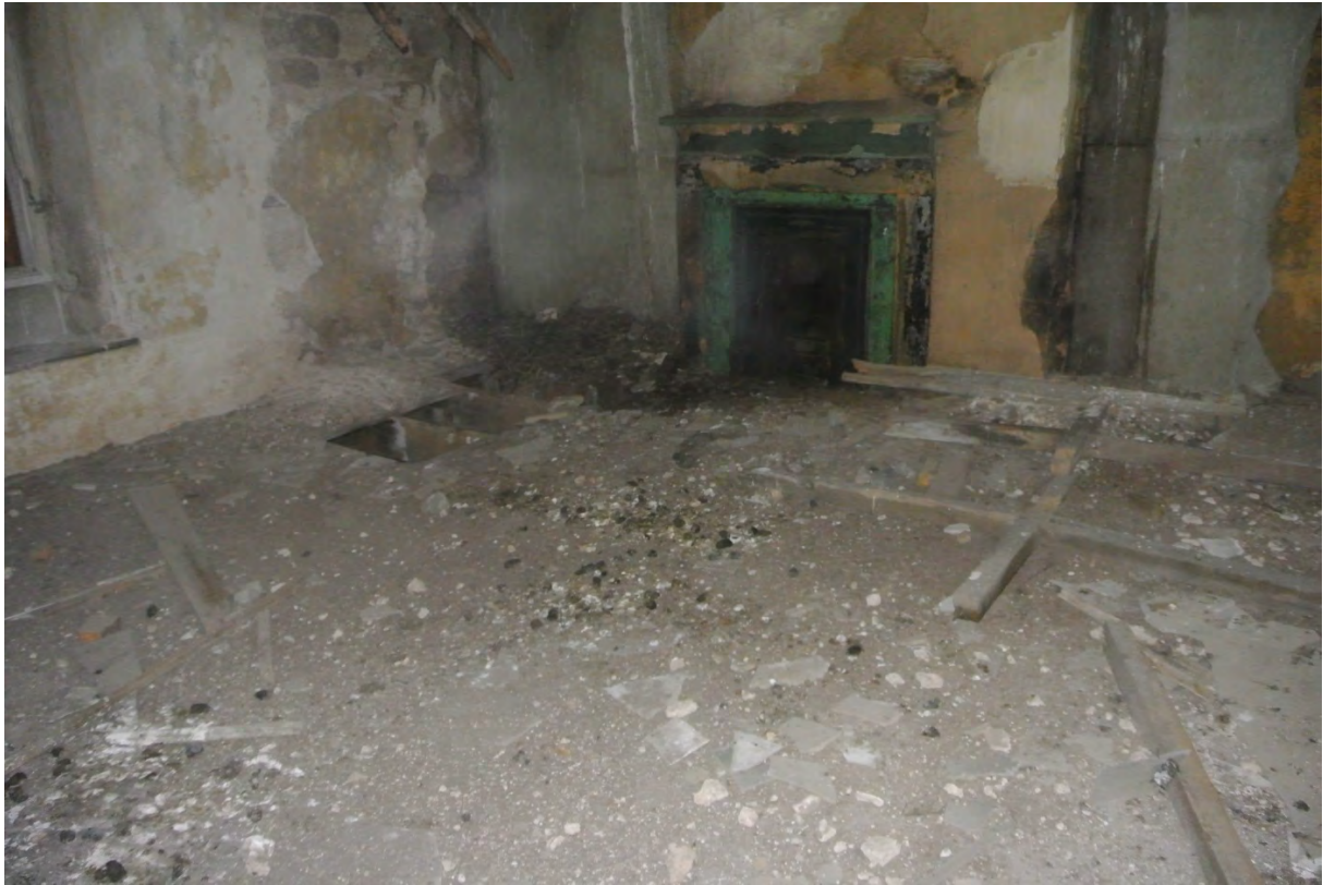
Internal view of West gable at first floor showing fireplace to be overhauled, fibre cement dry lining (ACM), rotten floor etc..
