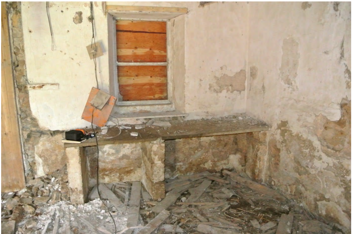
Closer view of stone shelf to removed / reused and existing window to be renewed.
