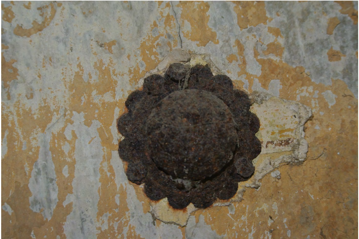
View of surface mounted “rosette” to be carefully removed and reused in refurbished building.
