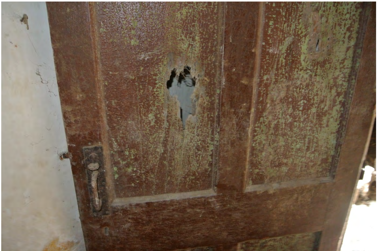
View of door to area 4 which is beyond repair
