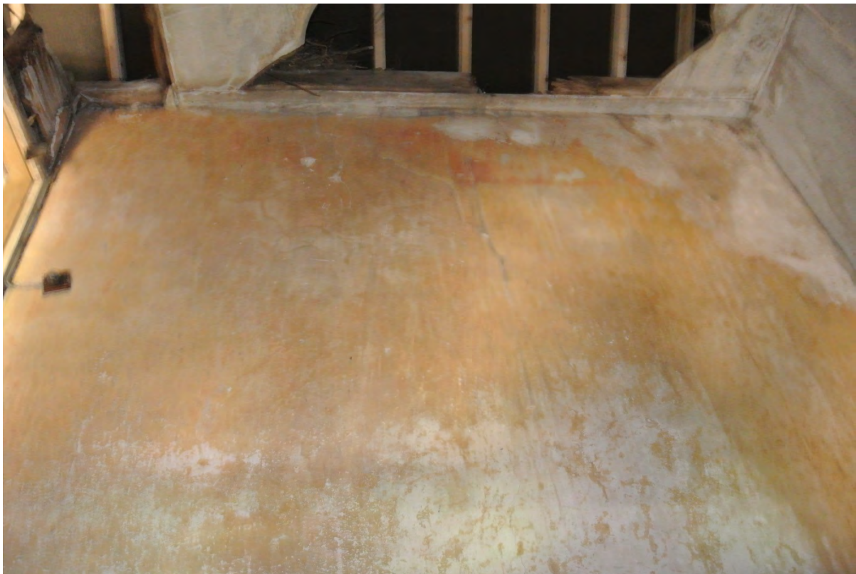
View of North wall in existing area 7 where new window to be formed for Bedroom 3. Fibre cement ceiling visible
