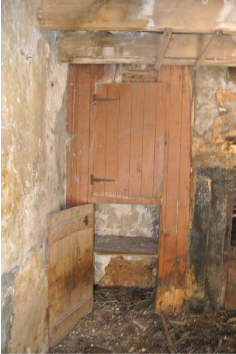
Detail of cupboard to be removed (LH side range) where new door to be formed to access extension
