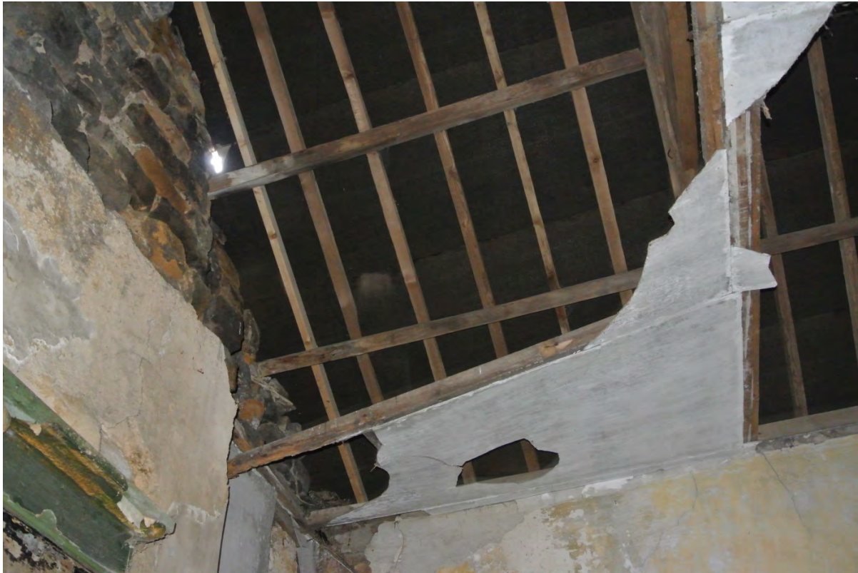
View of roof / fibre cement ceiling in existing area 6 where new rooflights to be installed.
