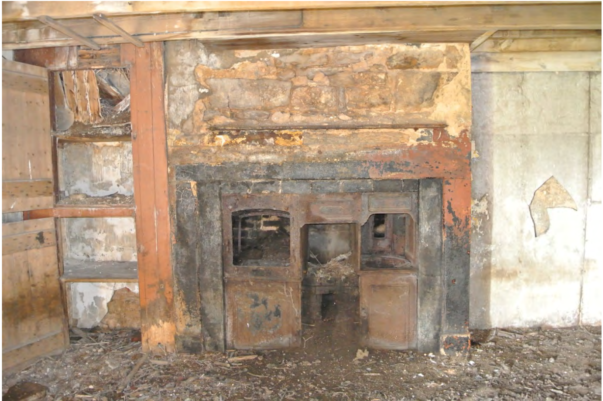
Closer view of range to be removed (decorative pieces to be retained and displayed in refurbished property)
