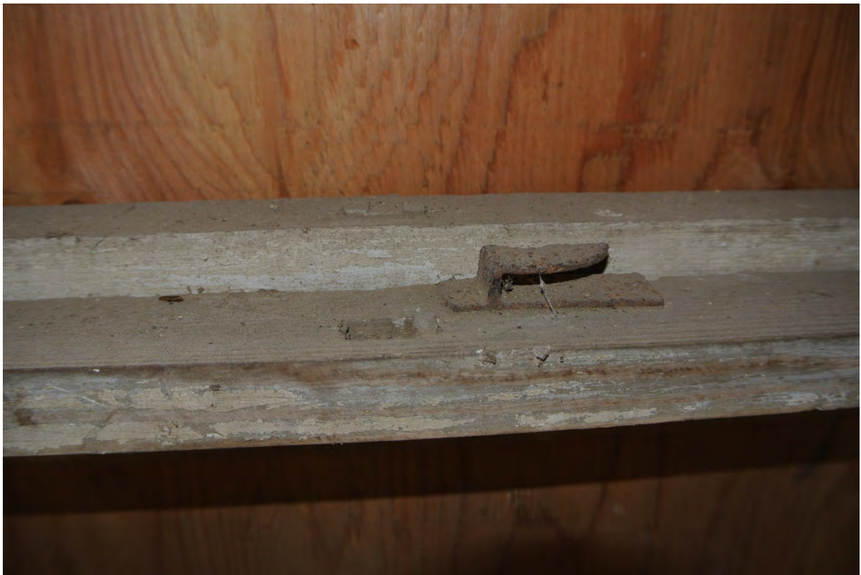
Detail of sliding sash window to South elevation in Area 1 showing mullion / glazing bar tenon hole
