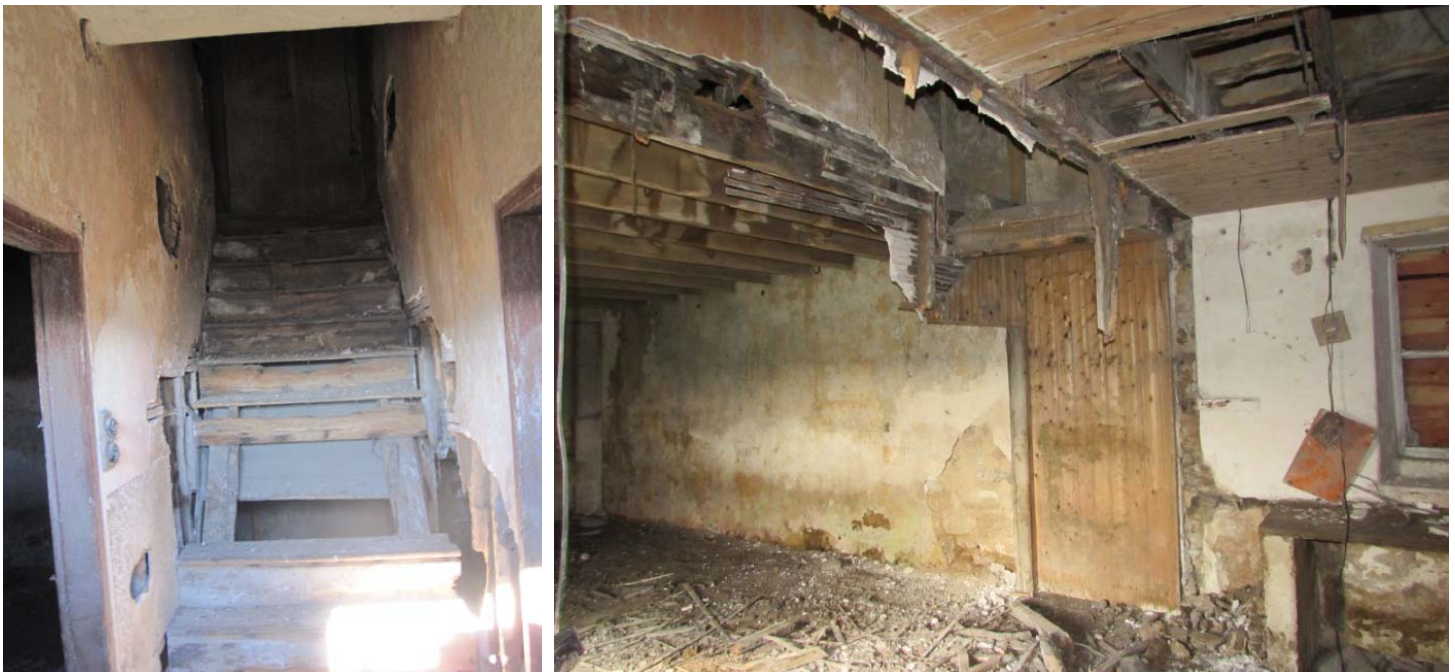
Fig.8 (left): 2012/2013 photograph showing former staircase and ground floor partition walls; (right): Current condition of cottage showing position of former staircase, as viewed Sept 2016
