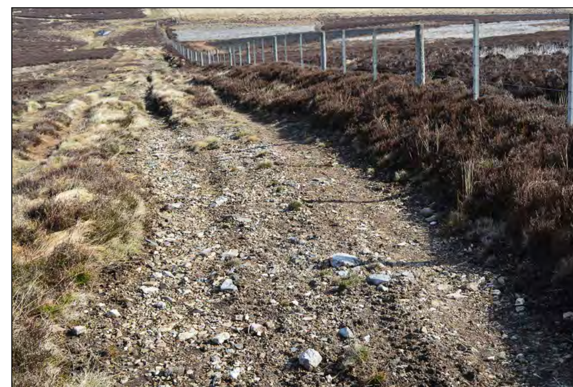
Track Deterioration Photograph (iii)
