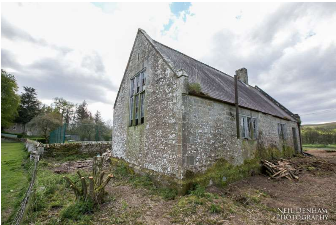
Plate 4. View towards the southern and eastern elevations. Note remnants of the original flue, the high level gable window, and the walled garden and tennis court to the west.
