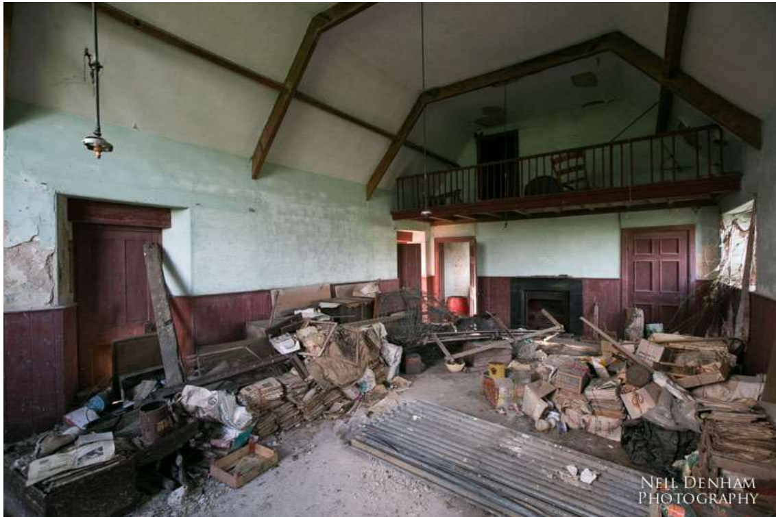
Plate 2. Internal view towards the mezzanine gallery. Note the open character of the space, and build-up of debris.
