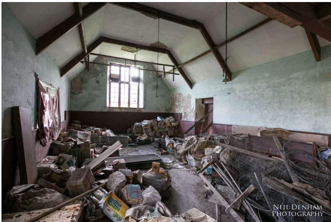
Plate 3. Internal view towards the southern gable. Note the high-level gable window, which is to be extended downward to facilitate external views from the new living space.
