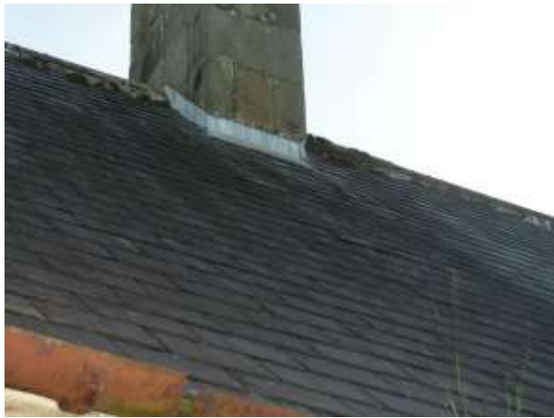
Chimney base with a few raised slates and crevices around, two Pipistrelle 45kHz bats emerged from this location
