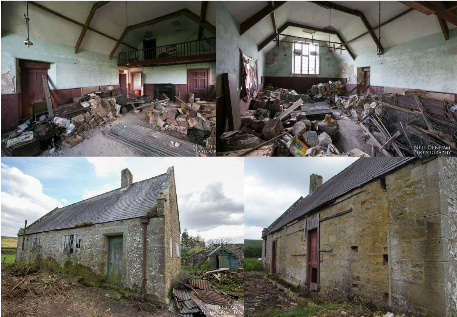
Internal and external images of building (extracts from D, A & H Statement) showing deteriorated condition
