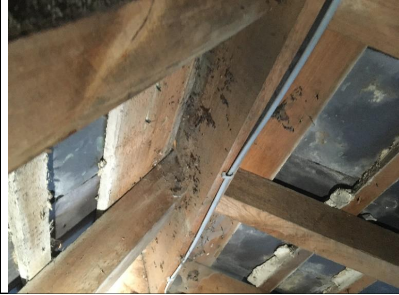
15. Bat droppings caught in cobwebs above loft hatch in centre of roof space
