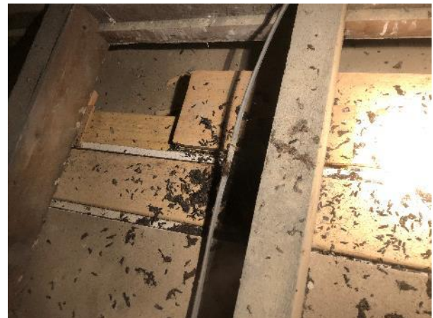
Mainly degraded pile of droppings, small number more recent
