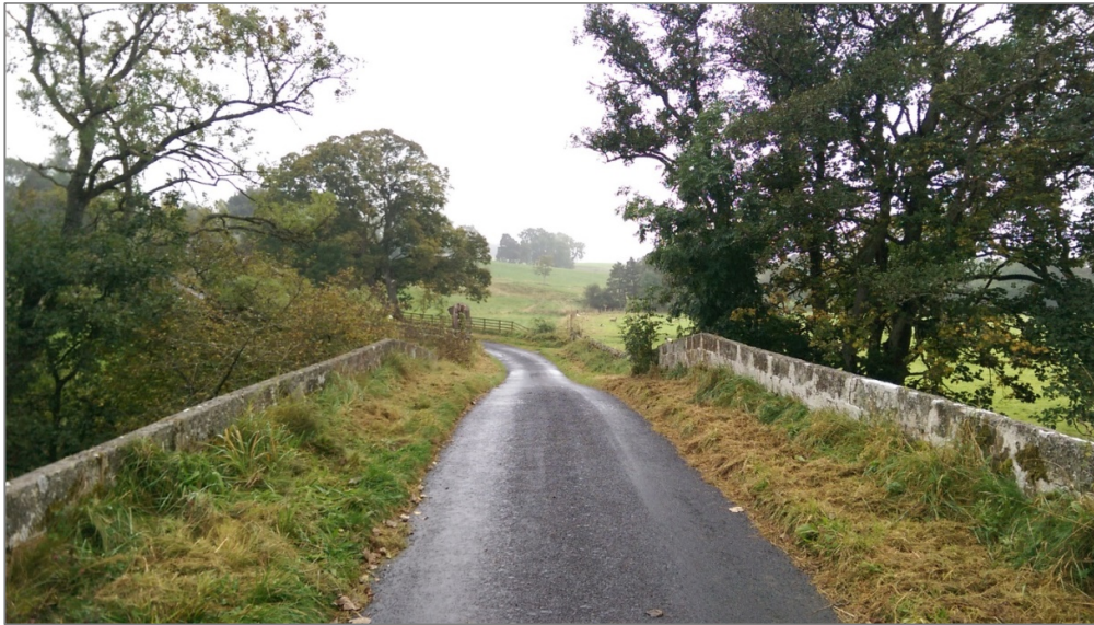
Photograph 1 – Poor surfacing and vegetation growth in verges looking southeast over bridge (16.10.2016)
