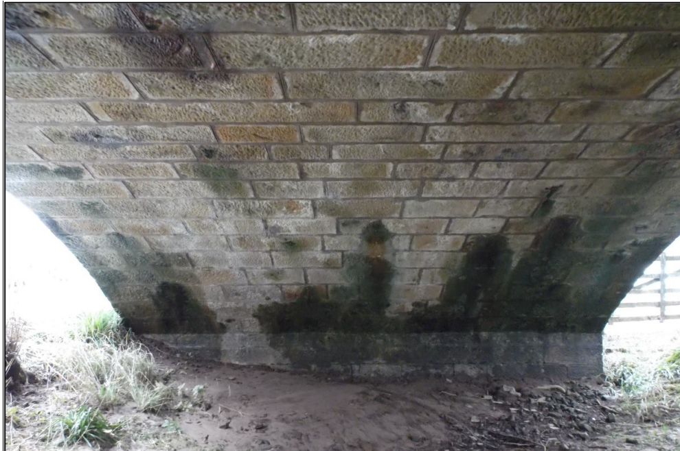
Photograph 2 – Dampness and staining to arch barrel masonry of north abutment
