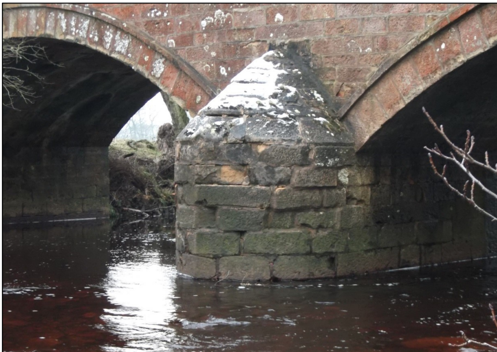
Photograph 9 – Open joints in east pier upstream cutwater, note evidence of recent spalling
