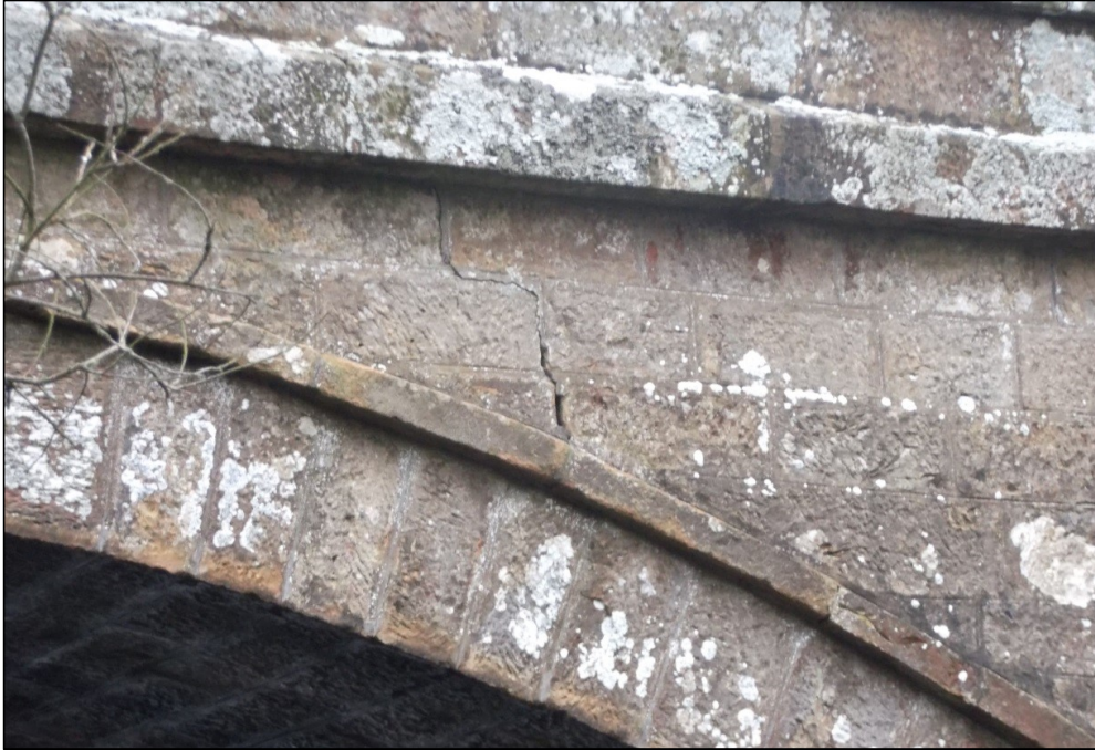
Photograph 5 – Crack in centre span spandrel to downstream elevation
