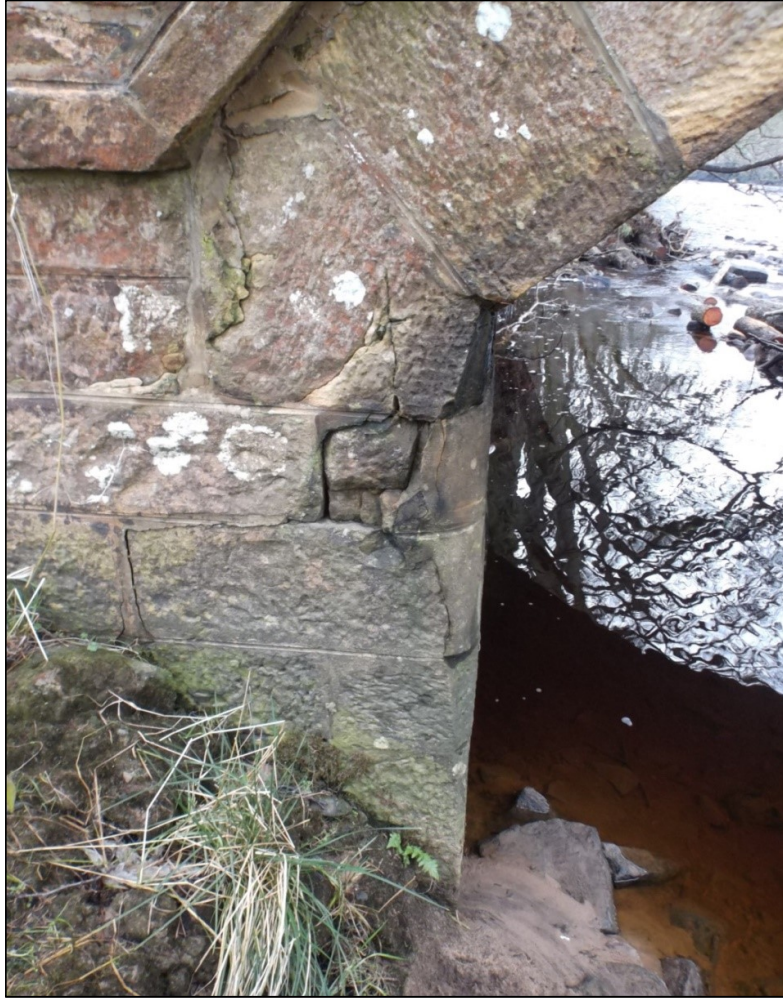
Photograph 7 – Masonry crushing at south abutment springing
