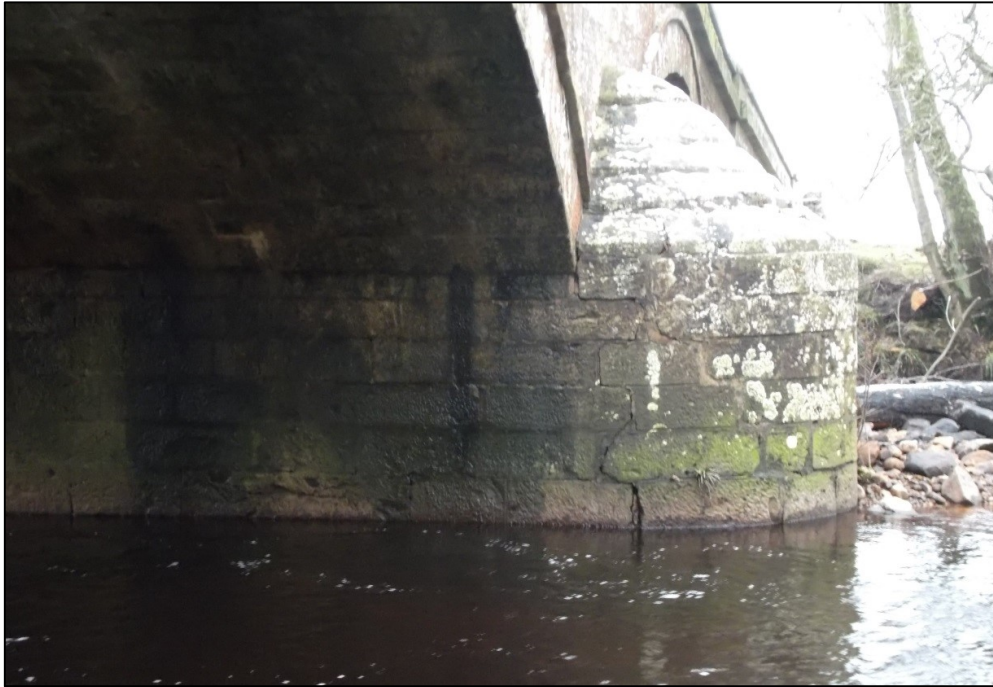
Photograph 8 – Crack and open joints to east pier downstream cutwater
