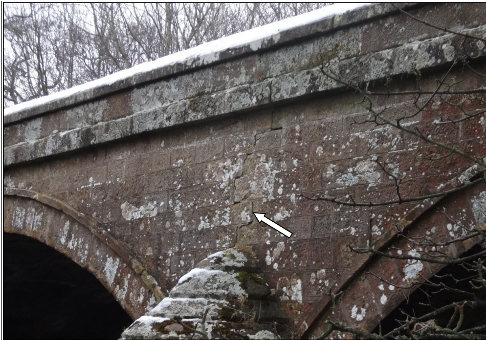
Photograph 4 – Crack above east pier to downstream elevation
