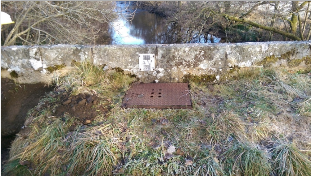
Photograph 11 – Abandoned water main cover to the Upstream verge (05/12/2016).
