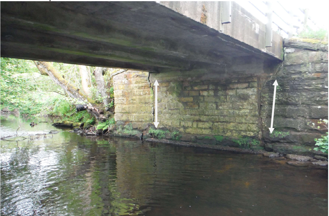
Photo 2 South abutment, arrows show cracks.
