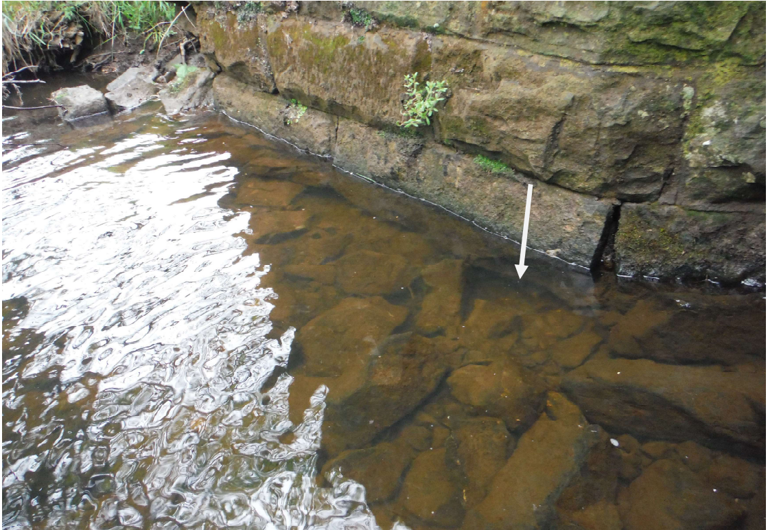
Photo 4 Scour area on west end of north abutment shown by arrow.
