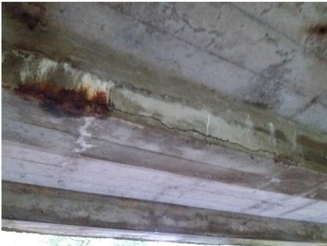
Figure 5 - View of longitudinal crack to downstand beam adjacent west elevation
