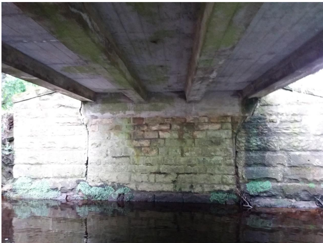
Figure 7 - Possible rotation of south wing walls
