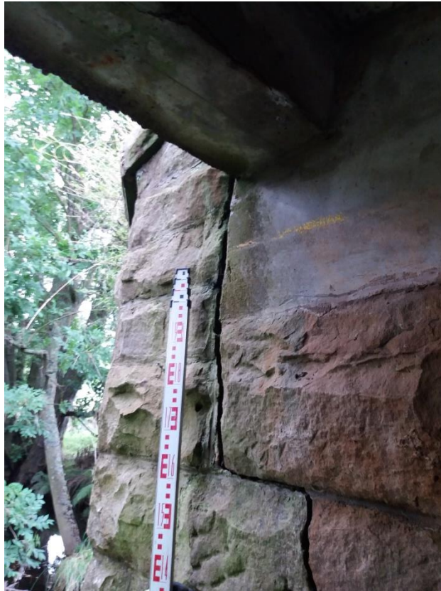
Figure 6 - Vertical step fracture at north abutment
