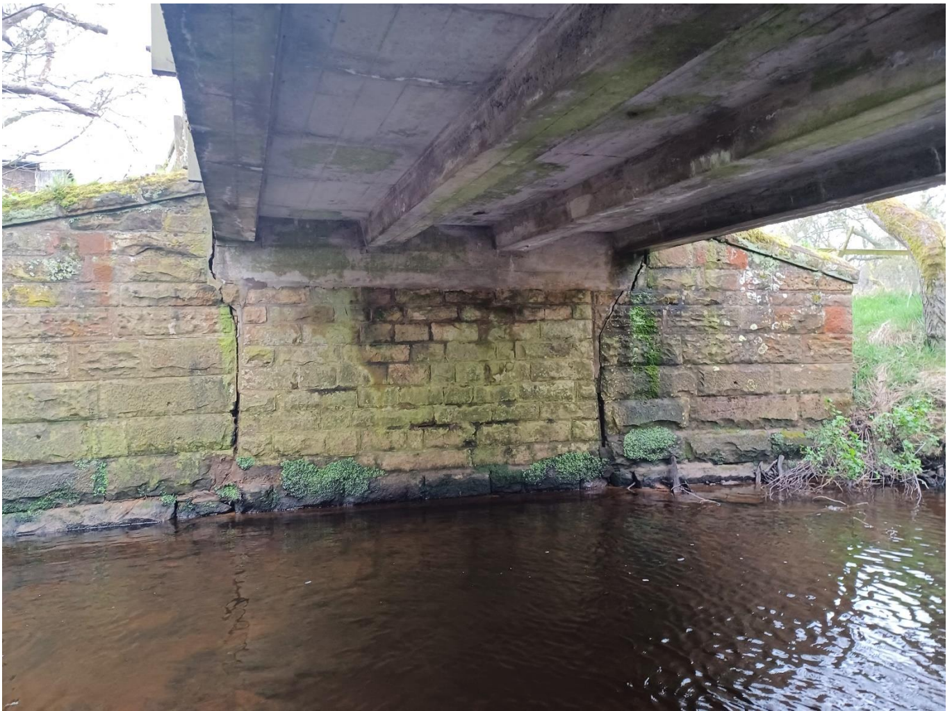
Figure 10. cracks in existing abutments and wingwalls (these will only be minimally impacted and gaps will be left in the masonry)
