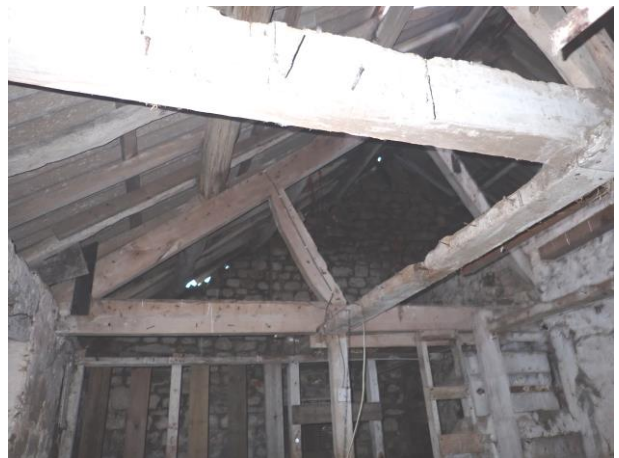
Gaps can be seen on west gable wall top, Barn Owl flew from this direction.
