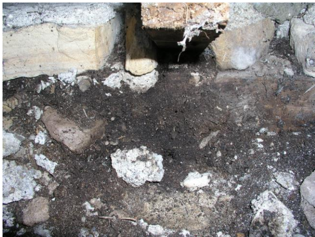
Photo showing disintegrated bat droppings beneath coping stones. If examined carefully, in the black dust exoskeletons of insects can be seen shining.
