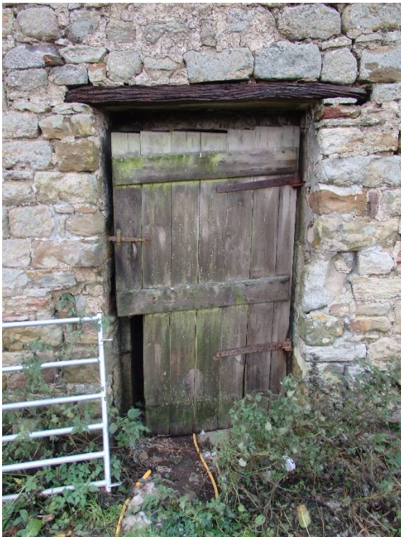
East elevation: Note displaced boards and poor condition of the door.
