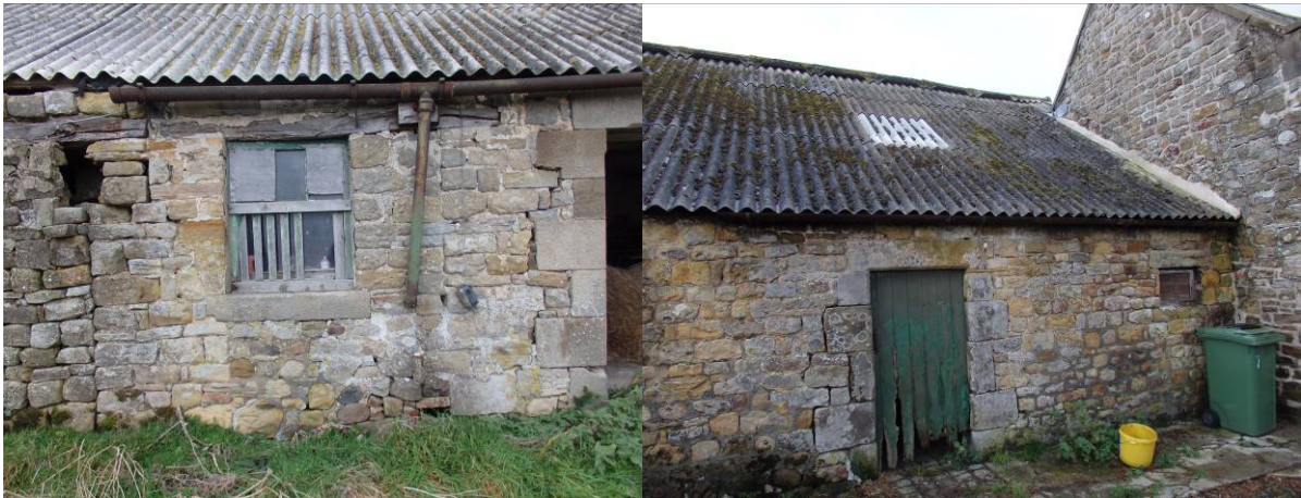
Southern elevation: Note the corroded and ineffective rainwater goods, the masonry panels of differing condition. Northern Elevation. Note the lack of guttering, and the poor condition of the door.
