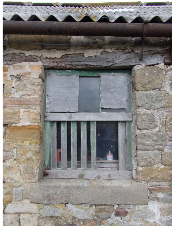
Southern Elevation. Note repairs to the traditional venting window with low level ventilation slats, partially missing.
