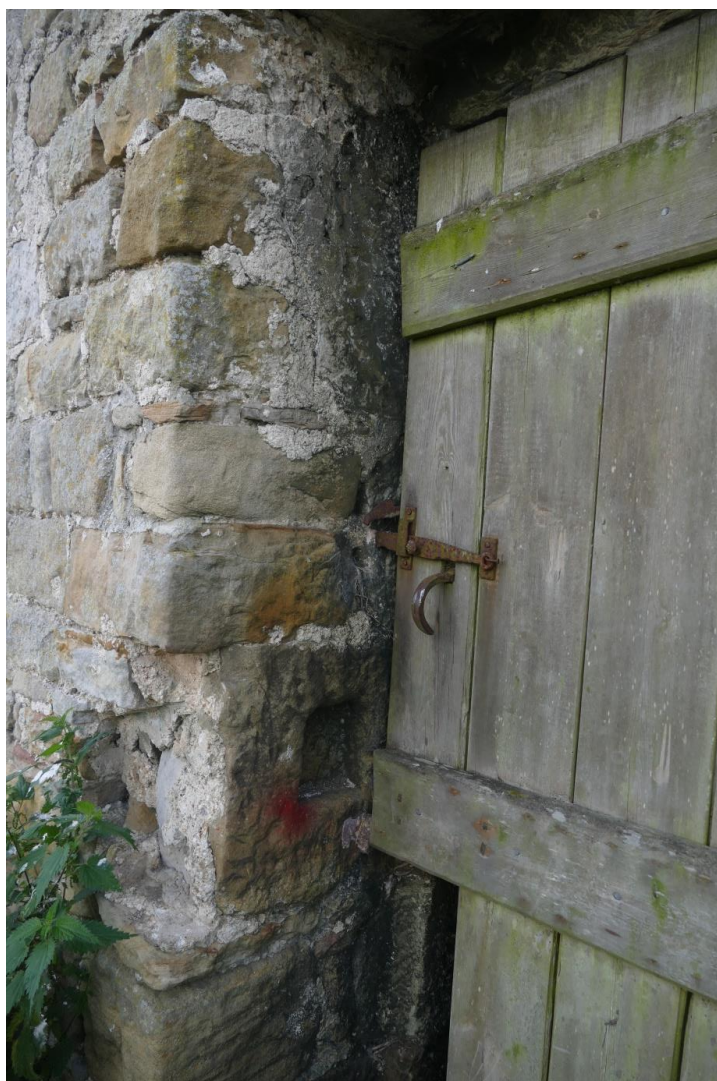
Doorway in East Wall, Inner (south) jamb, now external, with socket for draw bar
