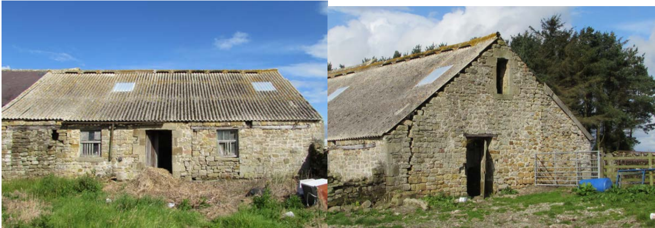
Figure 2: Southern (left) and eastern (right) elevations showing remnant rainwater goods and areas of failing stonework
