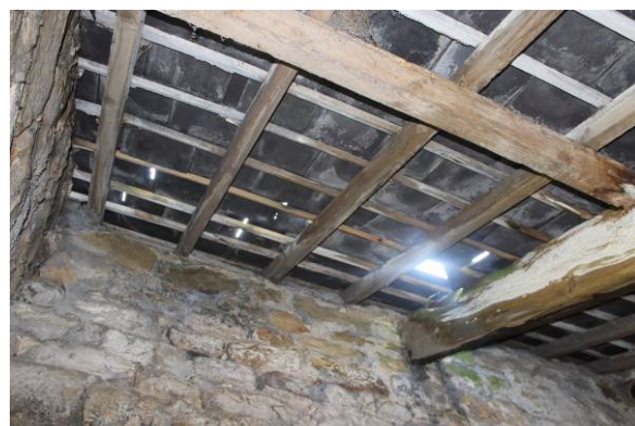
Kennel Roof. Note the missing and slipped slates, and decay to the purlin and principle rafter.
