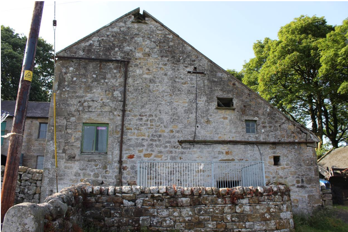
Southern Gable Wall. Note the missing stonework to the apex, the rainwater goods, and the displacement of the east kneeler and surrounding stonework.
