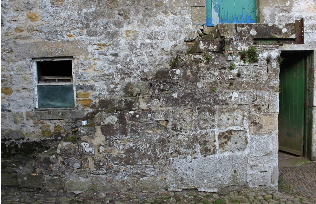
Western Elevation: Note the window with missing vertical glazing bars in a poor condition. Note the external stair is unprotected and is hazardous to use.
