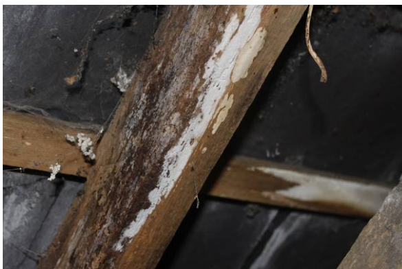
Store Roof. Note decay to one of the rafters.
