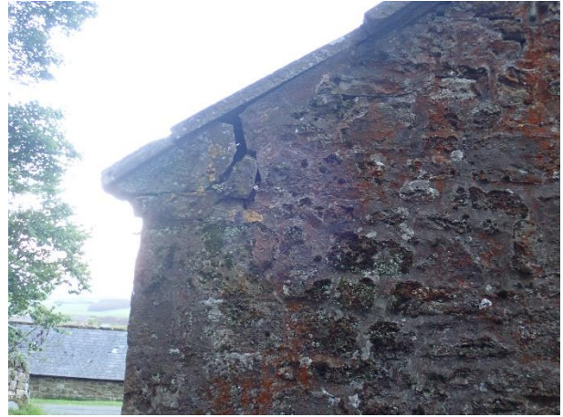
Missing apex, south gable
