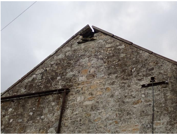
South gable crevices
