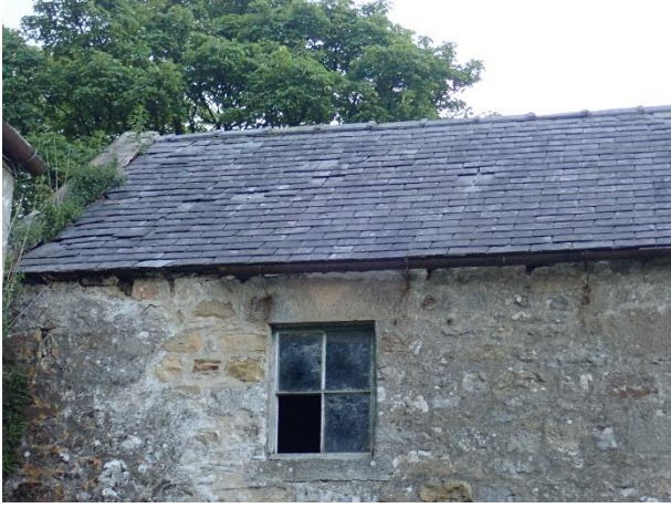
Roof with gappy slates
