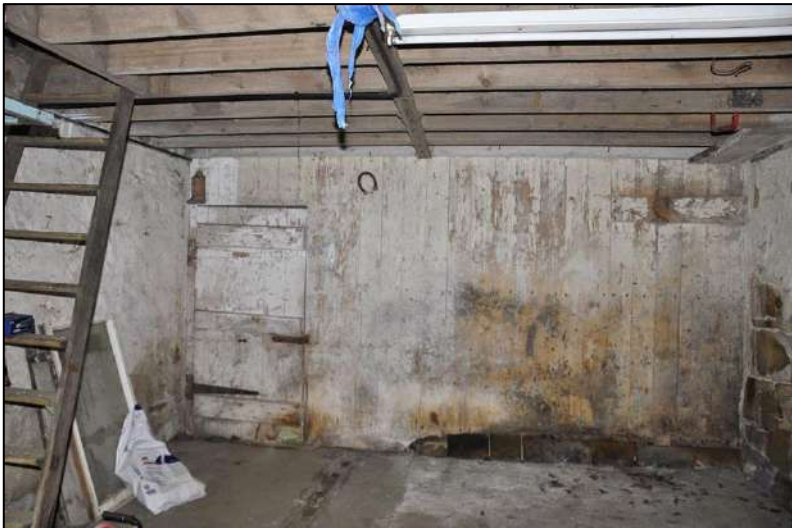
41. Original or early timber plank partition wall and door to later hay barn, south-east
