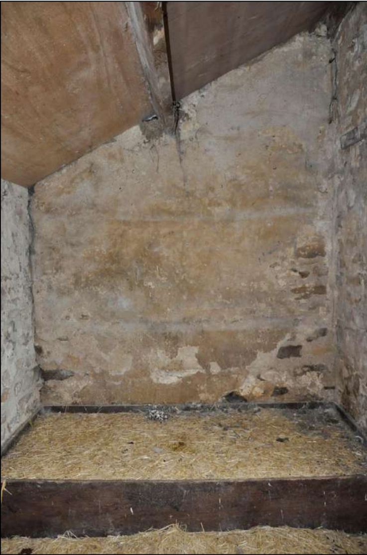
68. Internal view with modern timber kennel structure bed, lime plaster to rubblestone walls and modern concrete floor. Ceiling hidden above plyboard
