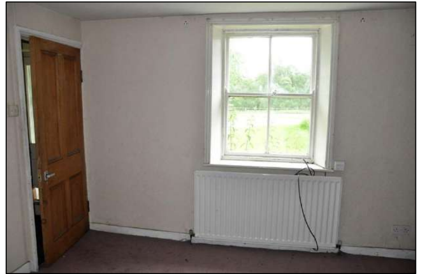
29. Four panel door with sash window. Modern skirting and radiator, front parlour
