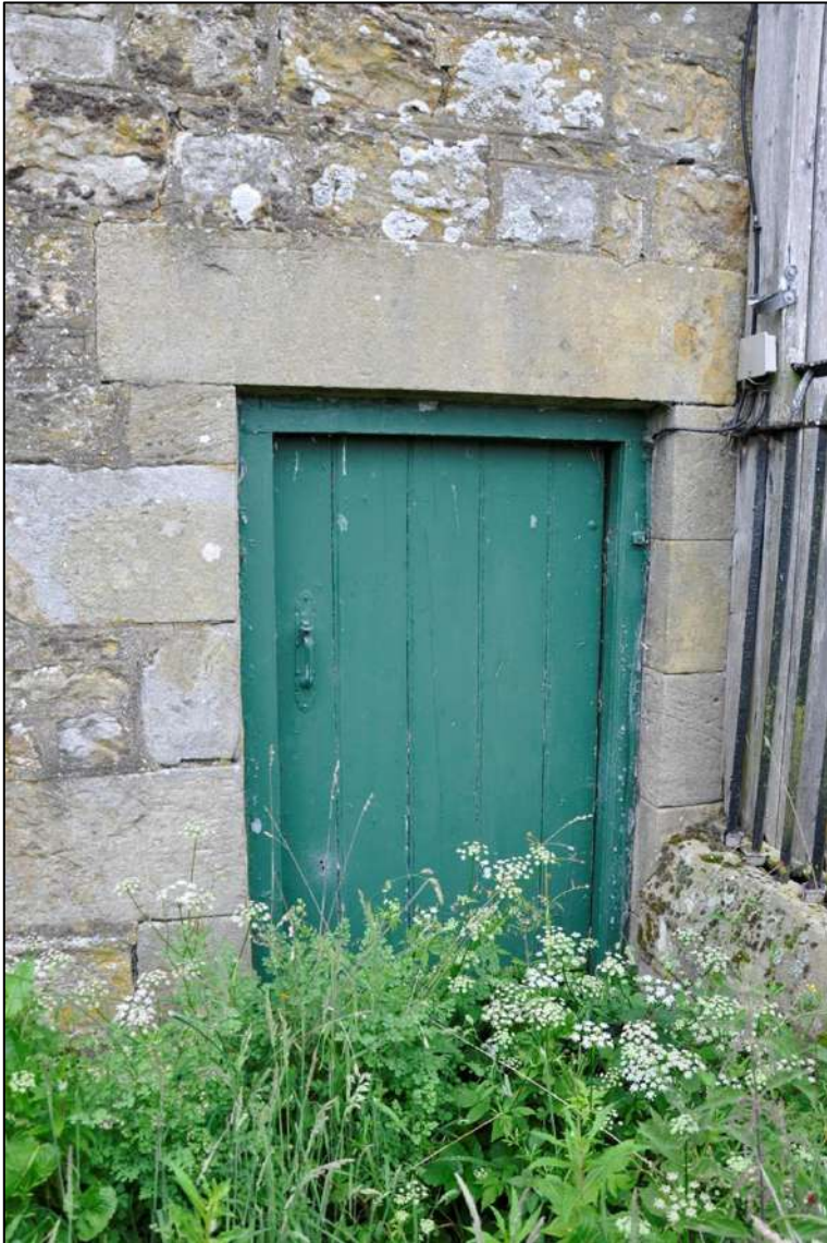
76. Entrance to boiler house with vertical plank door set in stone surround. Lintel not chamfered in contrast to original lintels
