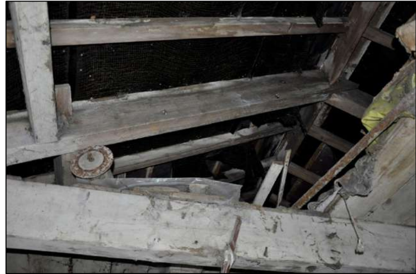
60. Dual pitched principal rafter roof structure, largely boarded with floorboards to create a small loft
