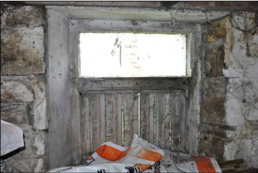
56. Internal view of window in plate 55. Note partially surviving timber reveals
