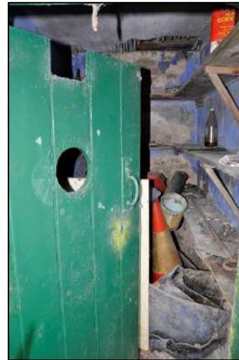
50. Detail of vertical boarded door to store with ventilation hole. Interior is lined with modern timber shelving with a partially exposed lathe and plaster ceiling
