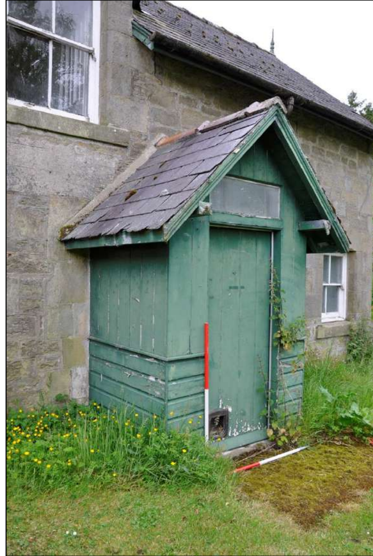
14. Detail of porch extension with original stone surround to original entrance opening visible (1m x 1m scales)
