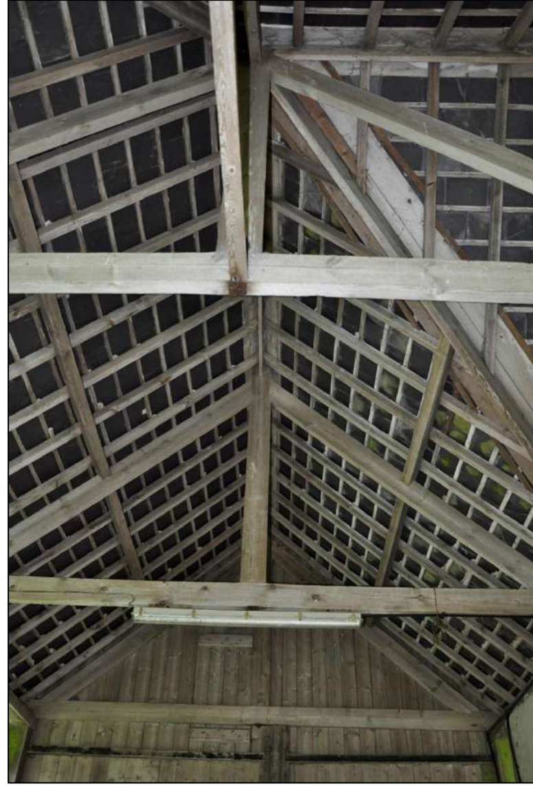
45. Detail of hay barn roof with king posts. Note redundant loft door to cart shed
