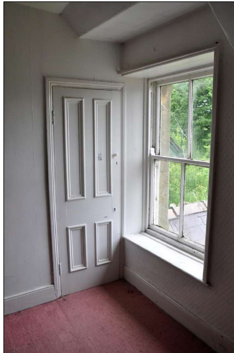
31. Four panelled cupboard door in moulded architrave, sash window, moulded skirting boards to front (eastern) bedroom
