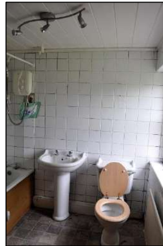
22. Modern bathroom subdivided a former larger ground floor room. Note timber boarded ceiling that continues across what is now the adjacent hallway
