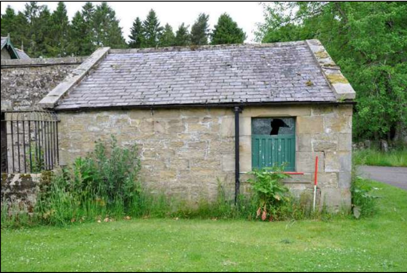
54. South-east elevation to stables with ventilated timber window (1m x 1m scale)
