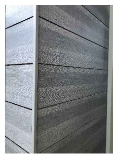
TRESPA CLADDING NATURAL MYSTIC CEDAR [PU 22] as installed on a recently completed project in Hexham and Corbridge
