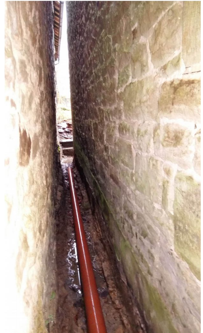
Area of stonework to be removed to the left of the photo to enable better access to Unit 3 and to reduce the risk of damp
