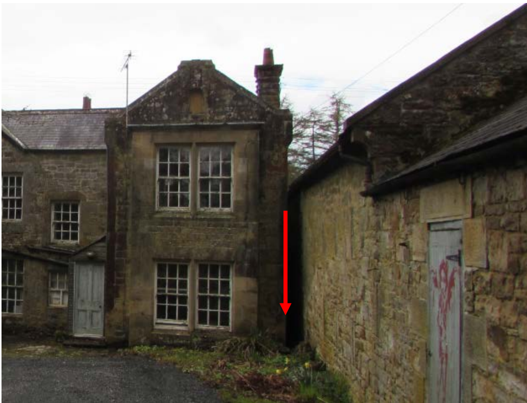
Figure 3: Photo showing gap between Unit 3 and the Dutch Barn
