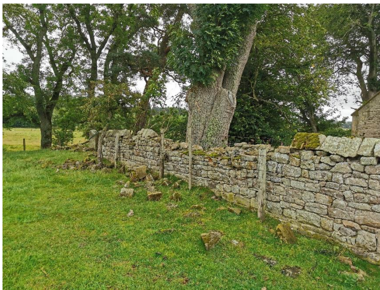
Photograph No. 10 - deterioration to northwest, low wall
