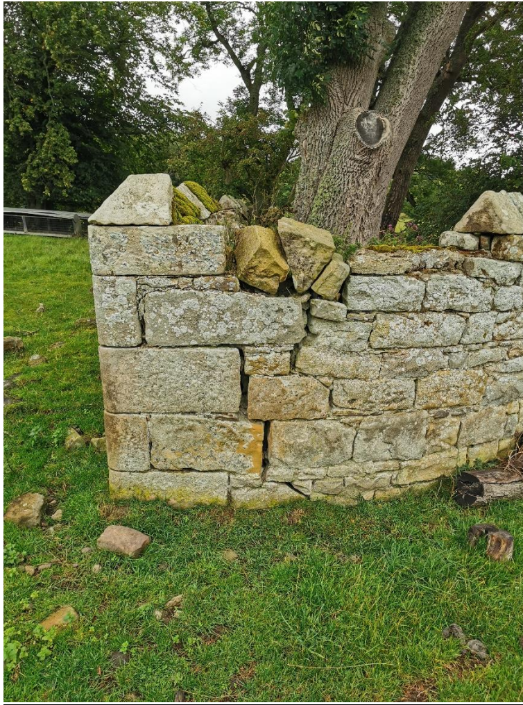
Photograph No. 9 – displacement of northwest, low wall
