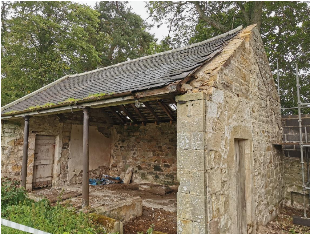
Photograph No. 6 – missing water table to central gable
