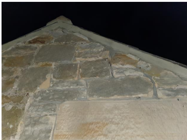
Gable end of log store from where a bat emerged. Crevice in the stonework above the lintel.
