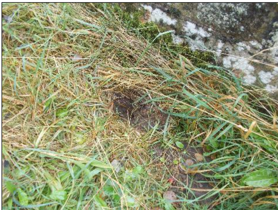
Image 7: Badger latrine on bridge
