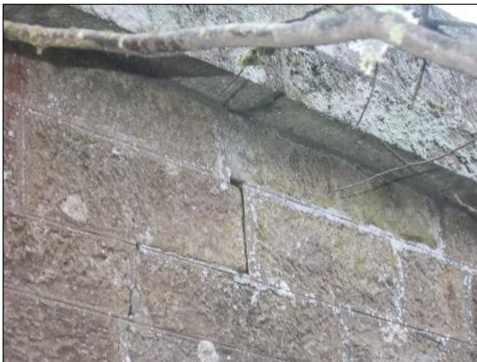
Image 3: Crack in the bridge stonework
