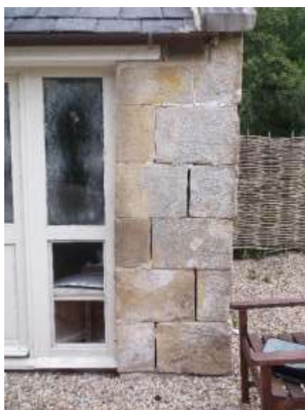
Photograph 6 – Misaligned quoin stones of western elevation.
