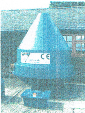
WPL Diamond DMS plant and kiosk with Alarm Beacon pictured right.
