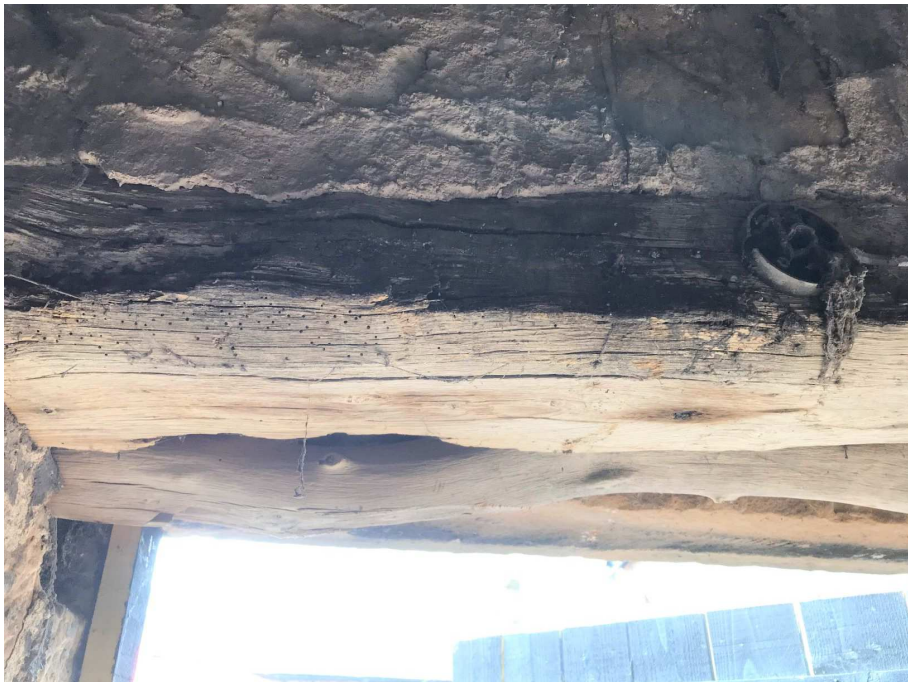
P12 – Minor woodworm flight holes to timber door lintels
