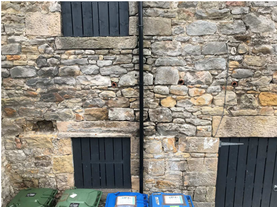
P8 – Open mortar joints to external walls
