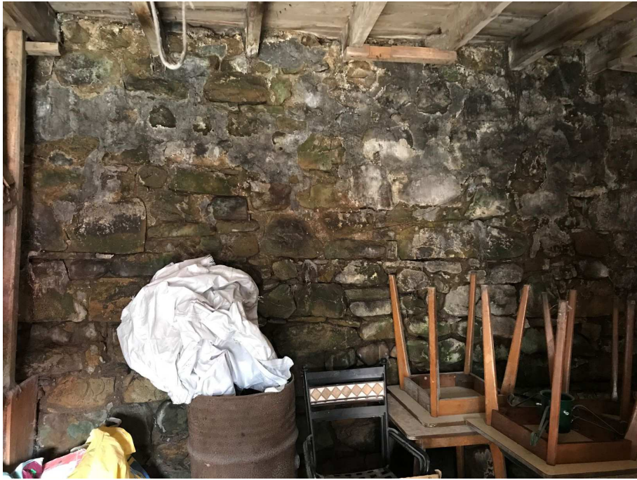
P11 – Algae growth / dampness to rear (north) retaining wall
