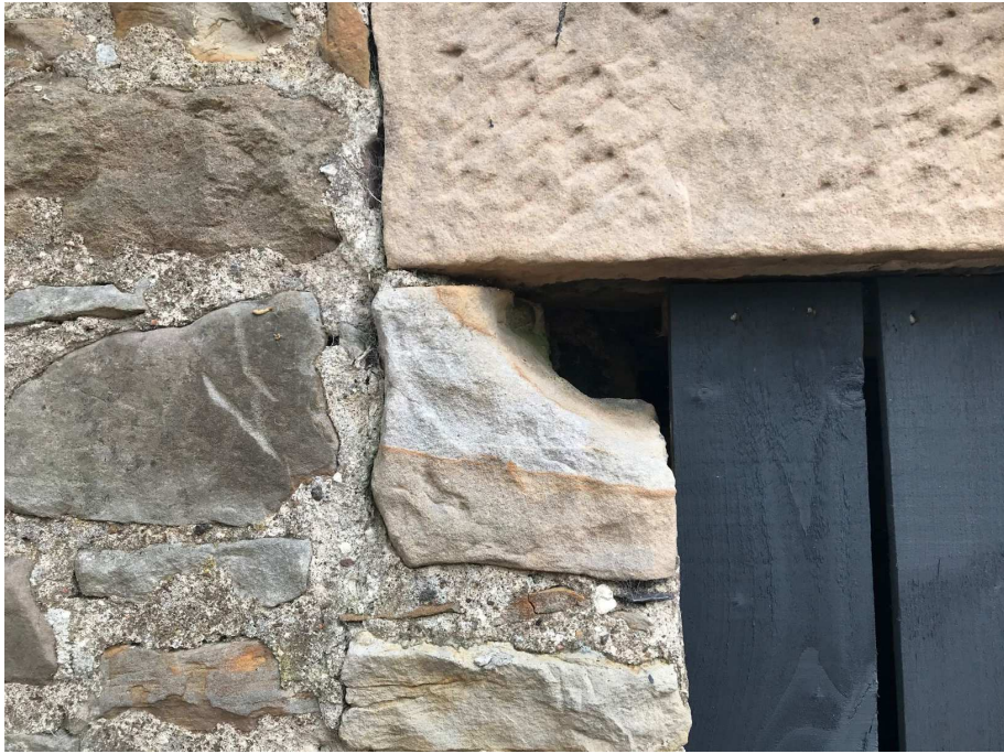
P7 – Eroded stone to west gable door jamb
