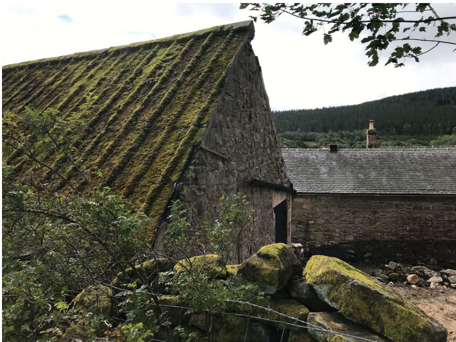
P4 – West gable wall / loose verge stones
