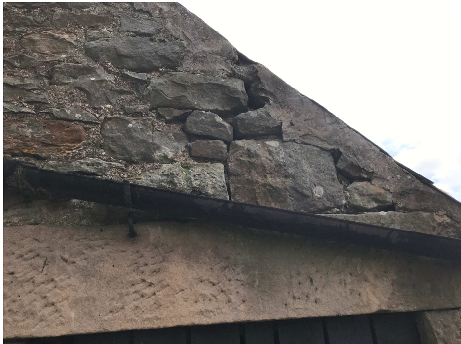
P6 – Loose stonework over west gable door opening
