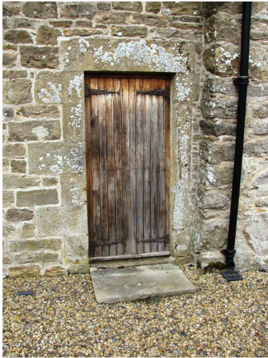
Existing 2016 entrance door to be replaced
