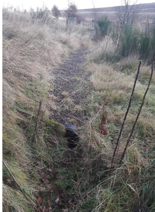
Ditch with last section covering large 18' pipe with gravel and pipe entering covered culvert
