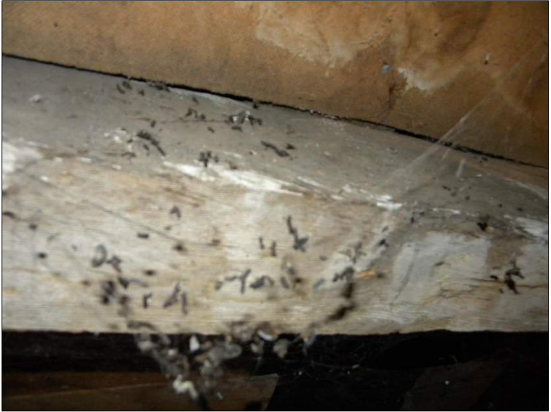
Figure 15. Bat droppings underneath MSD/OSB board to the south elevation pitch close to the chimney.
