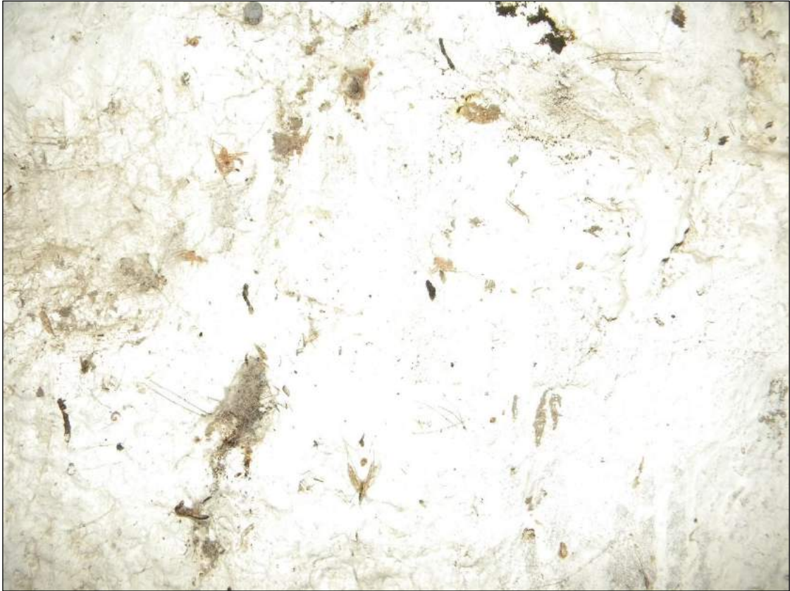
Figure 24. Bat and swallow droppings – west wall of stables adjoining the house
