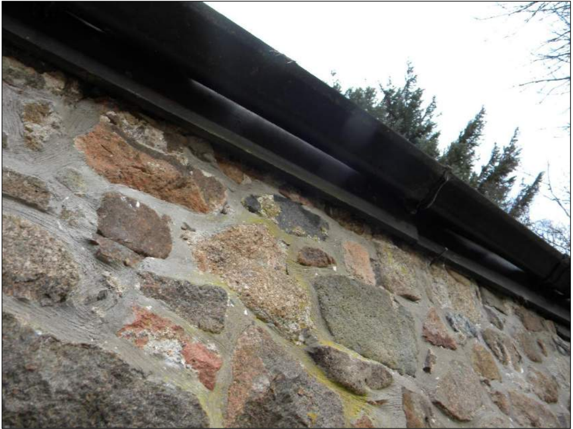
Figure 26. Building C. gaps under fascia
