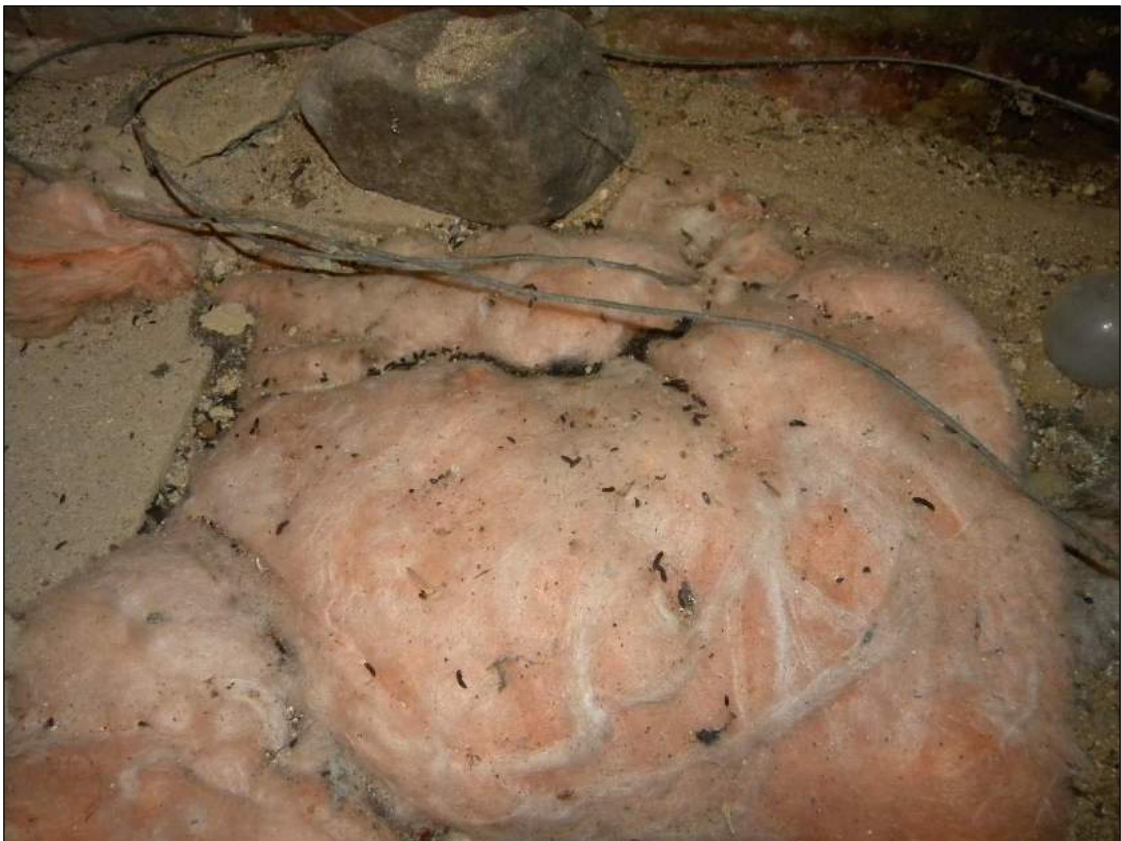
Figure 12. Bat droppings in loft below chimney
