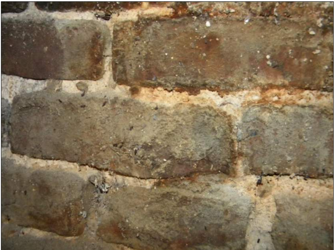
Figure 14. Bat Droppings on chimney flue in the loft.
