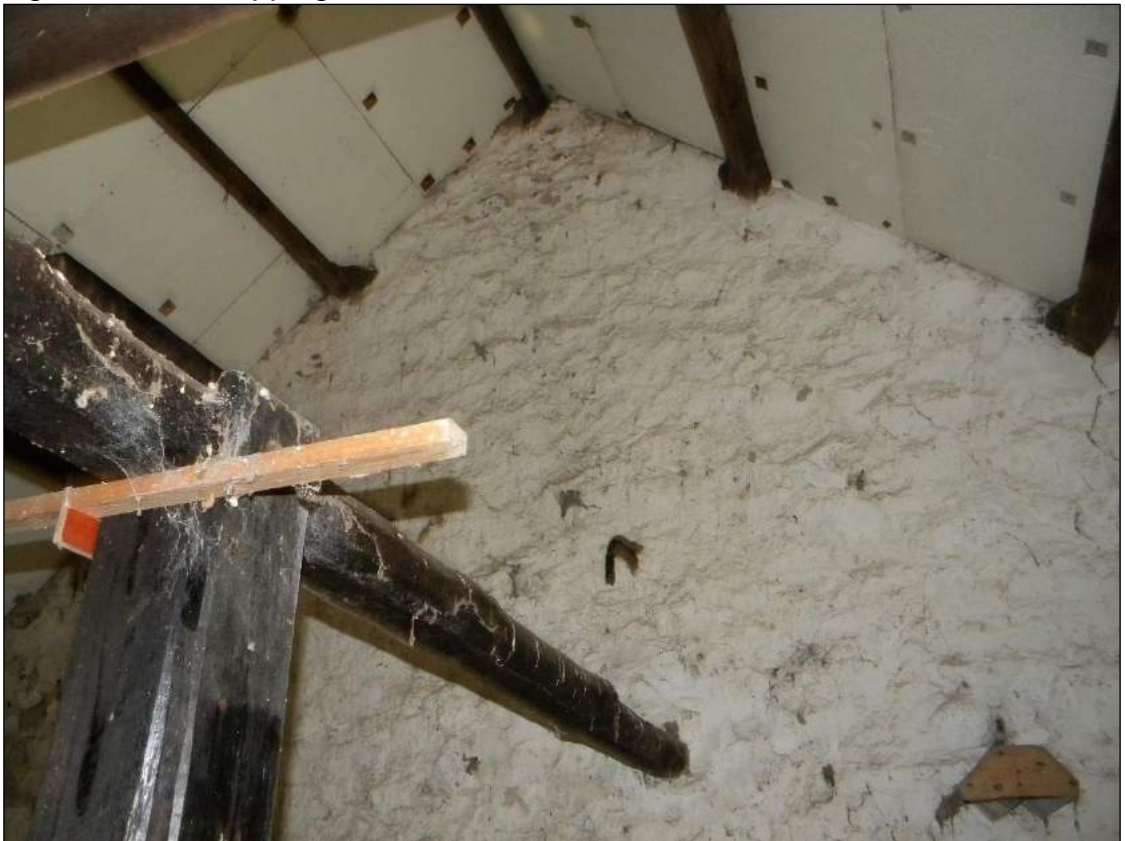
Figure 23. lined roof to the western section of the stables (adjoining the house).
