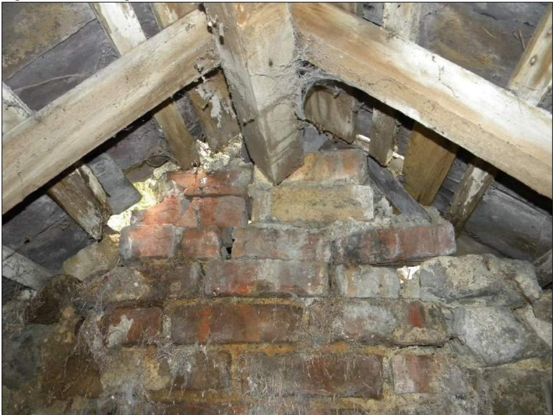
Figure 28. Building C. gaps to eastern gable in loft.
